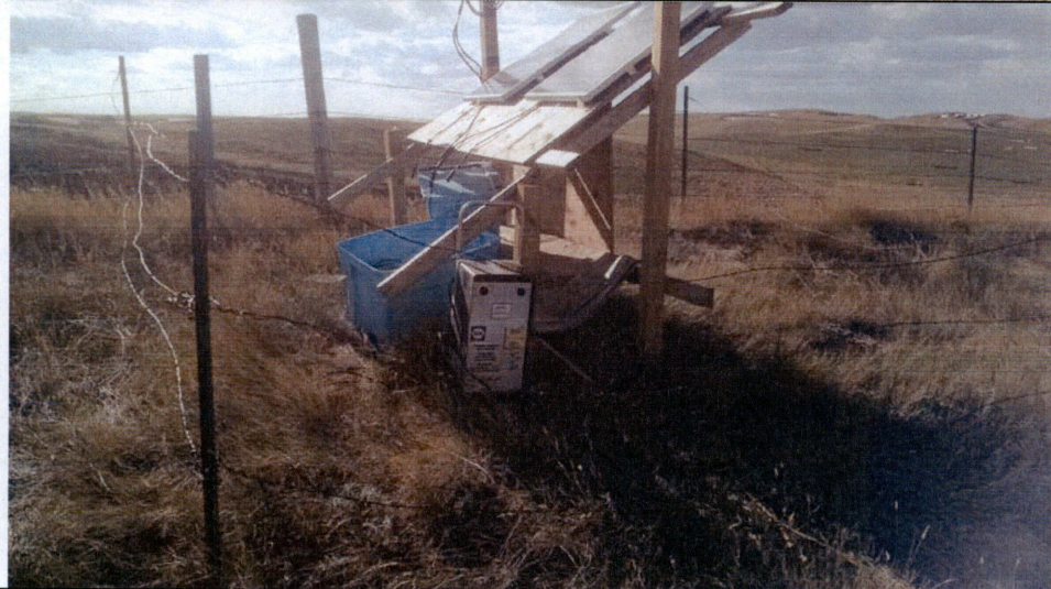
Photo 9: Temporary communication tower accidentally installed in cultural area, west of Turbine 19.
