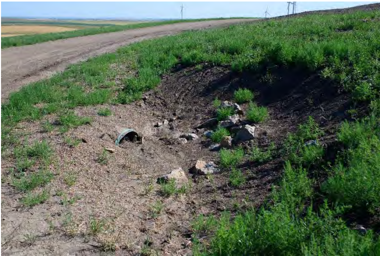
Photo 2: Between Tower 30 and 31 (facing North). Significant erosion, culvert filling with sediments (approximately 66% full)
