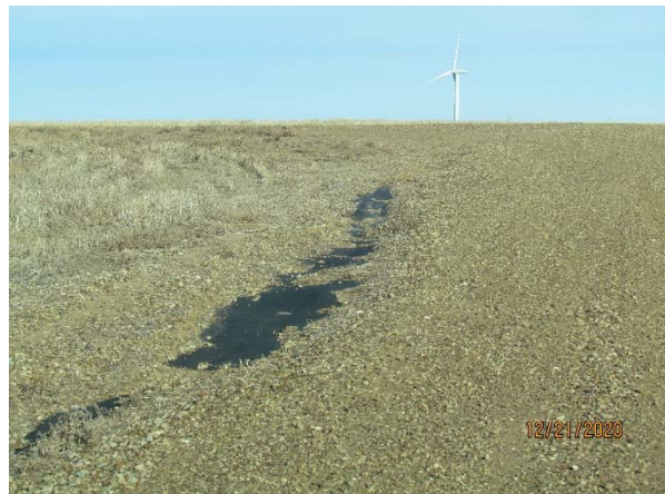
Photo 20: Exposed fabric near Turbine 5 at access road, facing north.
