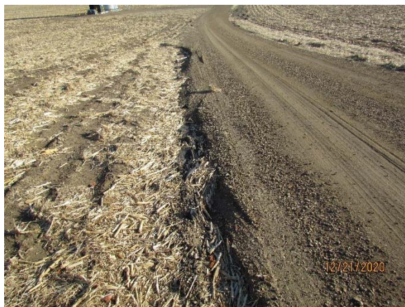
Photo 11: 10: Minor erosion on Turbine 2, 3, 4, 5 access road, facing east.
