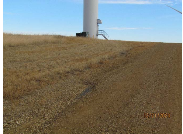
Photo 38: Minor erosion on access road near Turbine 12, facing east.
