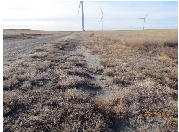
Photo 34: Minor erosion at access road near Turbine 9, facing southwest.
