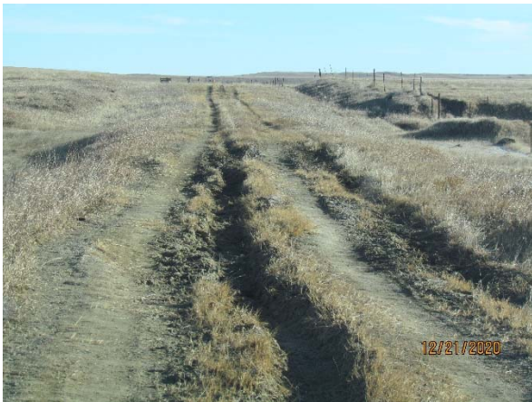
Photo 5: Section line (3 rd Avenue NE) roadway rutting, facing east.
