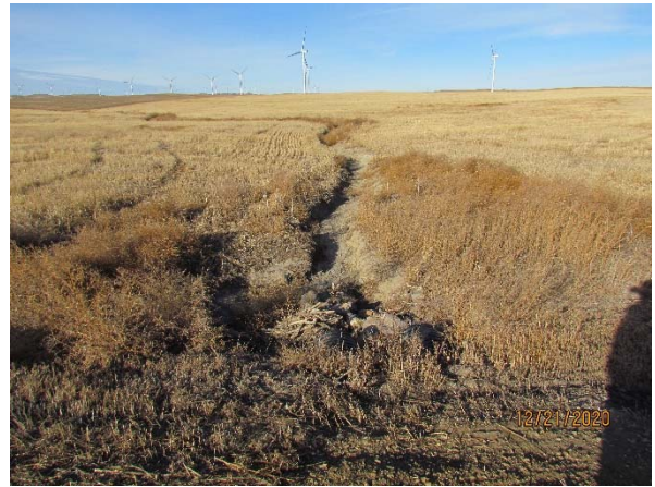
Photo 32: Access road (Turbine 6, 7, 8, 9) near Turbine 8, access road erosion, facing west.
