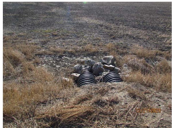
Photo 30: Access road (Turbine 6, 7, 8, 9) culvert, minor erosion and sedimentation, facing northwest.
