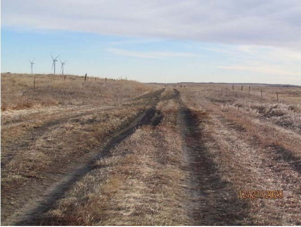
Photo 1: Section line (3 rd Avenue NE) roadway rutting, facing east.
