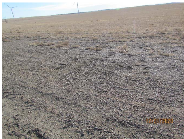
Photo 23: Settling of access road near Turbine 1, facing south.
