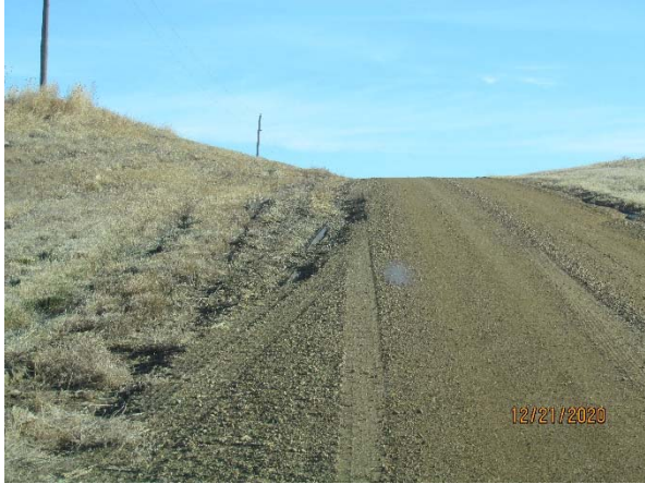
Photo 25: Minor erosion on North side of access road, facing east
