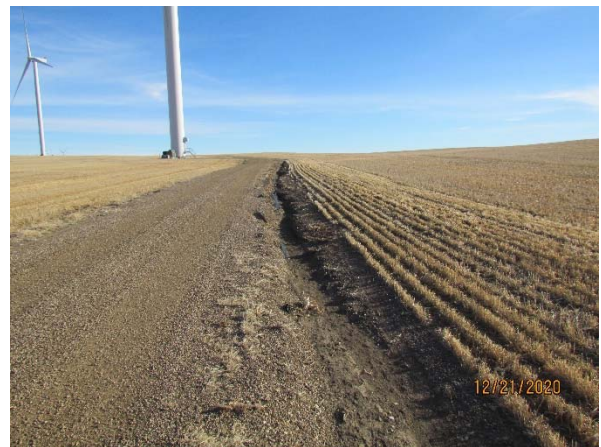
Photo 16: Erosion near Turbine 3, facing east.
