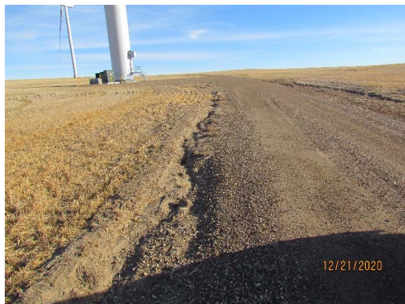
Photo 17: Erosion near Turbine 3, north side of access road, facing east.
