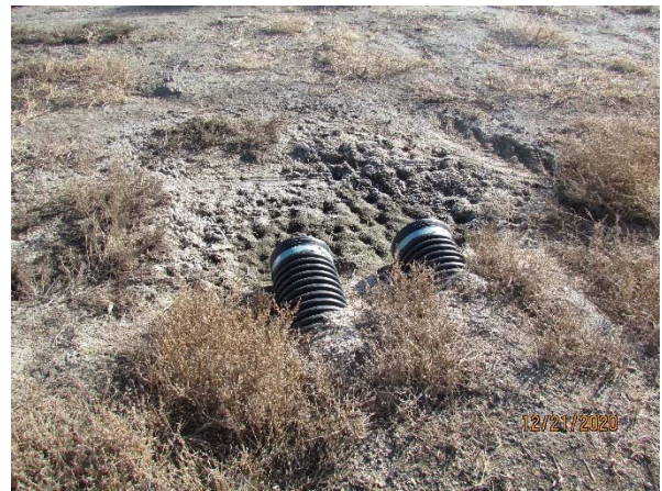
Photo 36: Access road near Turbine 9, erosion and sedimentation at culvert crossing, facing east.
