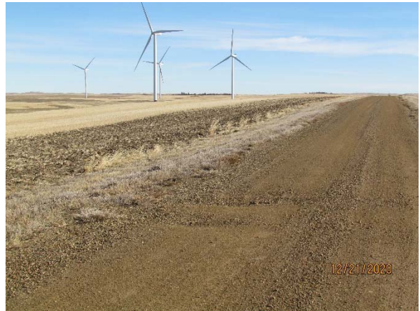
Photo 26: Settling / pothole on north side of access road, facing east.
