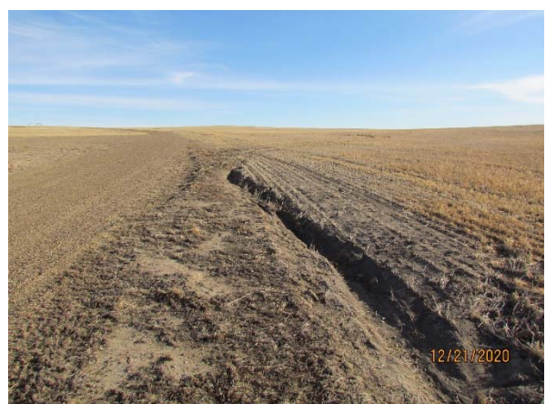
Photo 18: Erosion near Turbine 3, south side of access road facing east.
