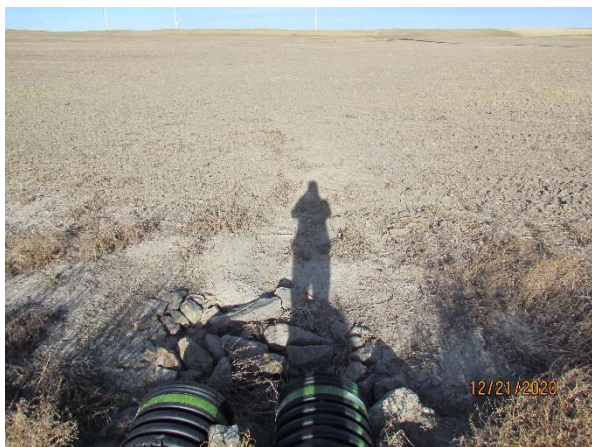
Photo 29: 7 th Street NE (near Turbine 6, 7, 8, 9 access road) culvert, minor erosion and sedimentation (south)
