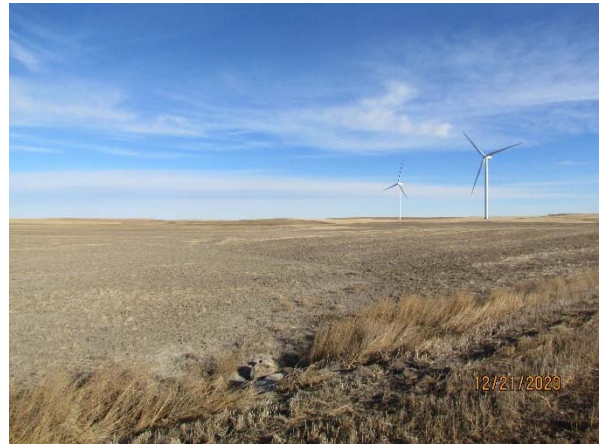
Photo 28: 7 th Street NE (near Turbine 6, 7, 8, 9 access road) culvert, minor erosion and sedimentation at waterbody crossing, facing north.
