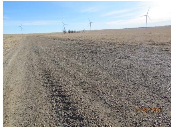
Photo 22: Settling of access road near Turbine 1, facing south.
