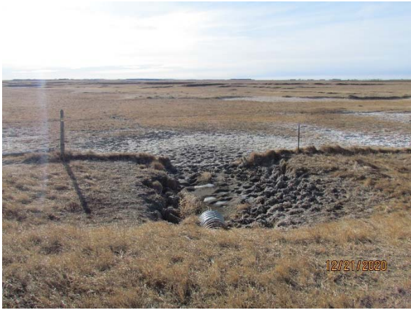
Photo 7: 3 rd Avenue NE crossing culverts and erosion, facing south.
