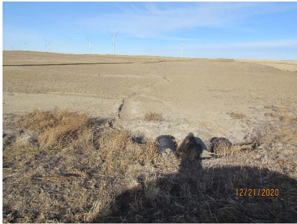
Photo 31: Access road (Turbine 6, 7, 8, 9) culvert, minor erosion and sedimentation, facing southeast.
