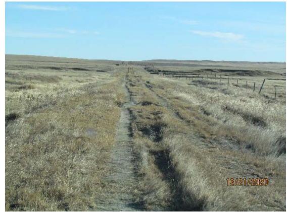
Photo 4: Section line (3 rd Avenue NE) roadway rutting, facing east.
