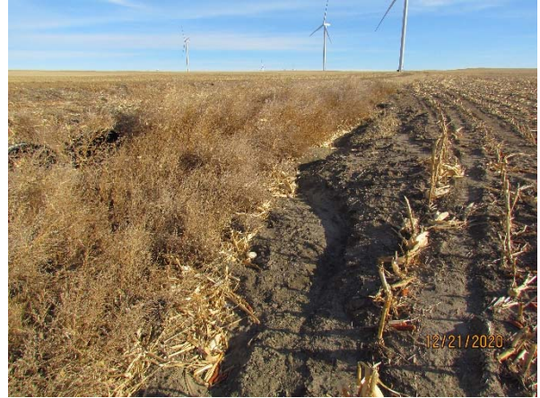
Photo 14: Erosion on Turbine 2, 3, 4, 5 access road, facing east.
