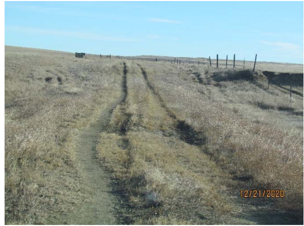
Photo 8: Section line (3 rd Avenue NE) roadway rutting, facing east.
