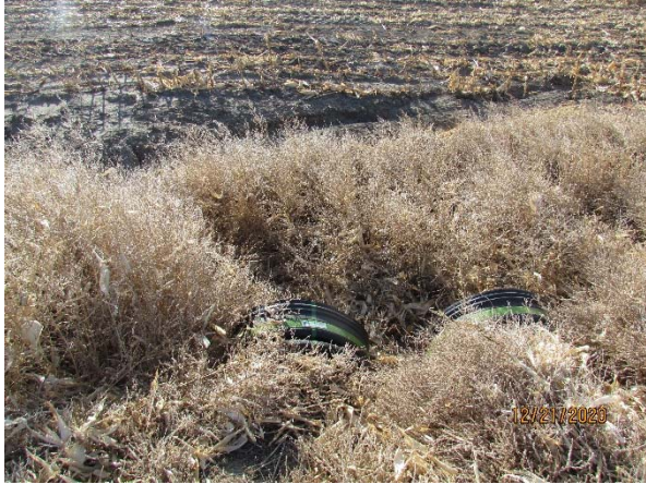
Photo 13: Waterbody crossing and minor erosion on Turbine 2, 3, 4, 5 access road, facing south.
