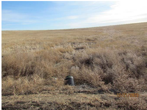
Photo 33: Access road erosion near Turbine 8, access road, facing east.
