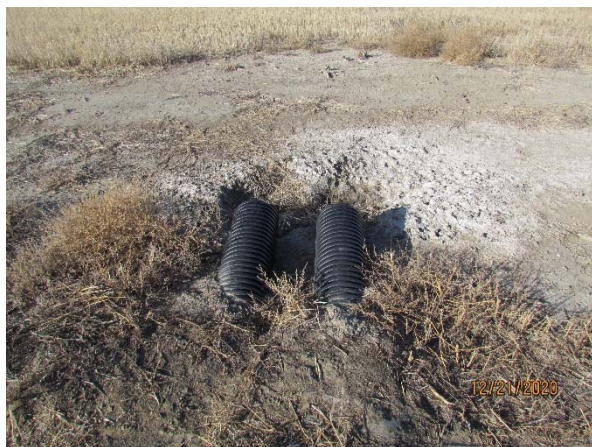
Photo 35: Access road near Turbine 9, erosion and sedimentation at culvert crossing, facing west.
