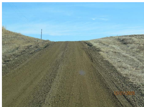
Photo 24: Minor erosion on North side of access road, facing east.
