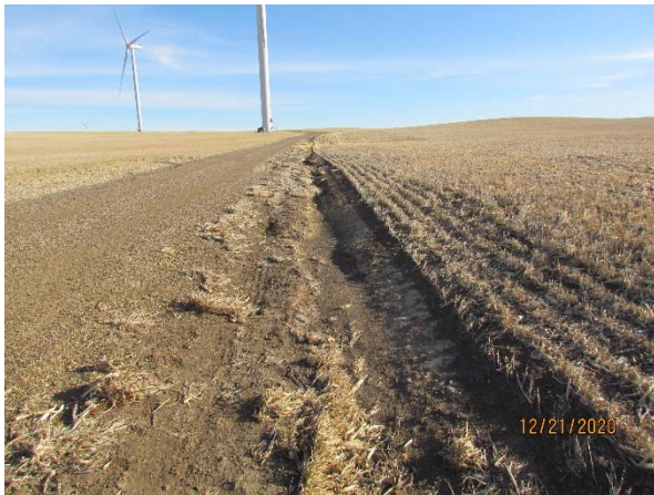
Photo 15: Erosion on Turbine 2, 3, 4, 5 access road, facing east.
