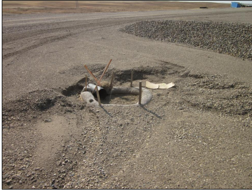
Photo 9. Direction: Northeast. Drain line surrounded by straw wattles to prevent sediment from entering the drainage.
