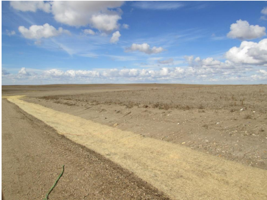
Photo 8. Direction: East. Fiber blanket placed in a ditch to control erosion and sediment migration along the northern edge of the project area.
