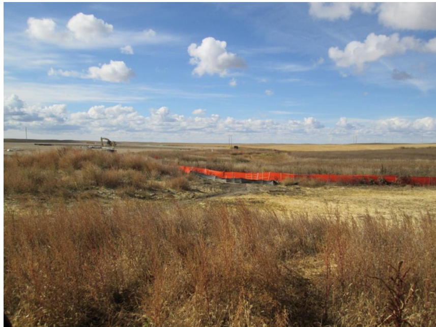
Photo 10. Direction: West. Silt fences in place around a wetland installed to prevent sedimentation.
