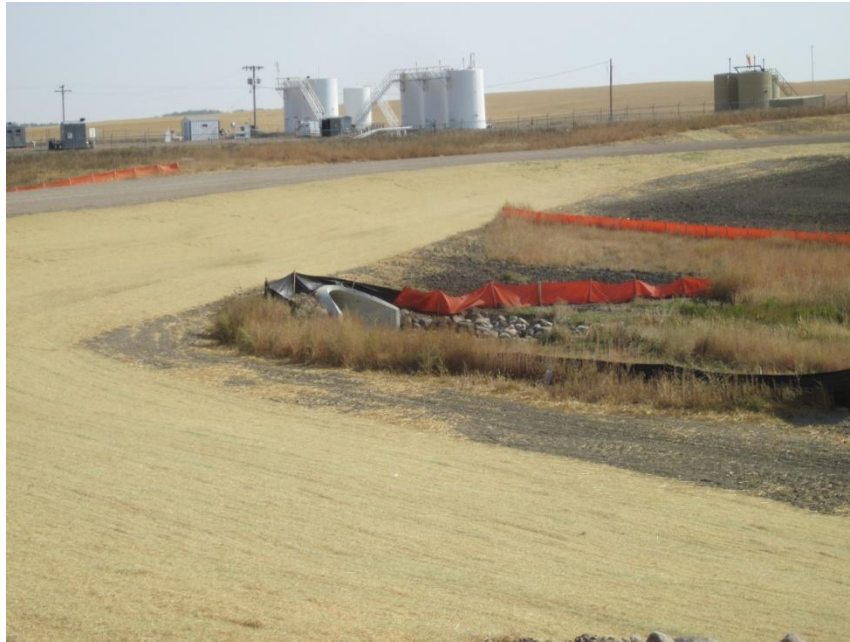
Photo 13. Direction: East. Culvert surrounded by rip-rap and silt fences to prevent sedimentation.
