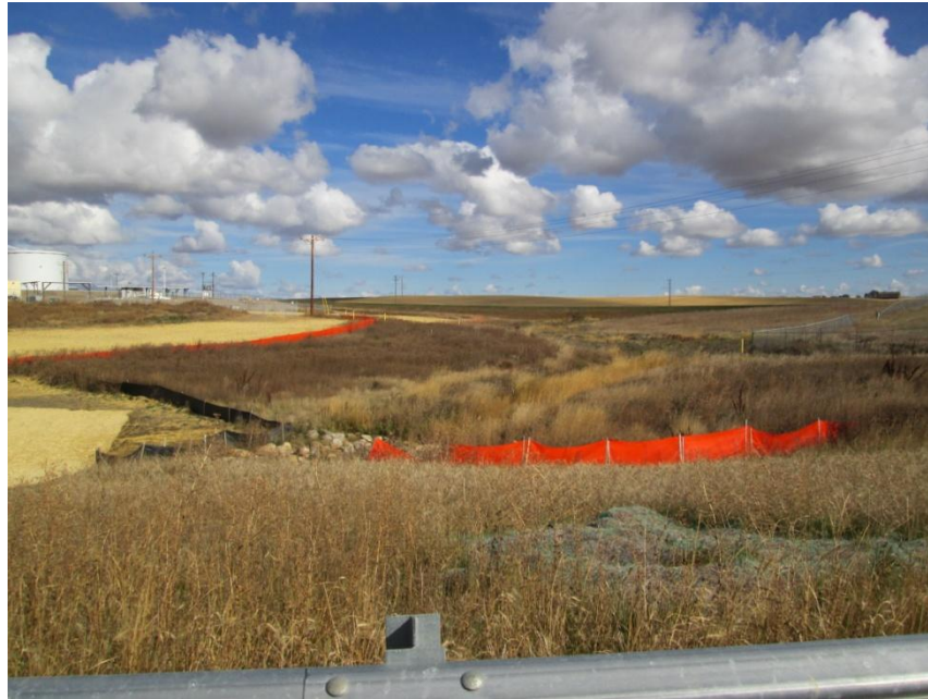
Photo 11. Direction: East. Silt fences and rip-rap around a drainage to protect the wetland for sedimentation.
