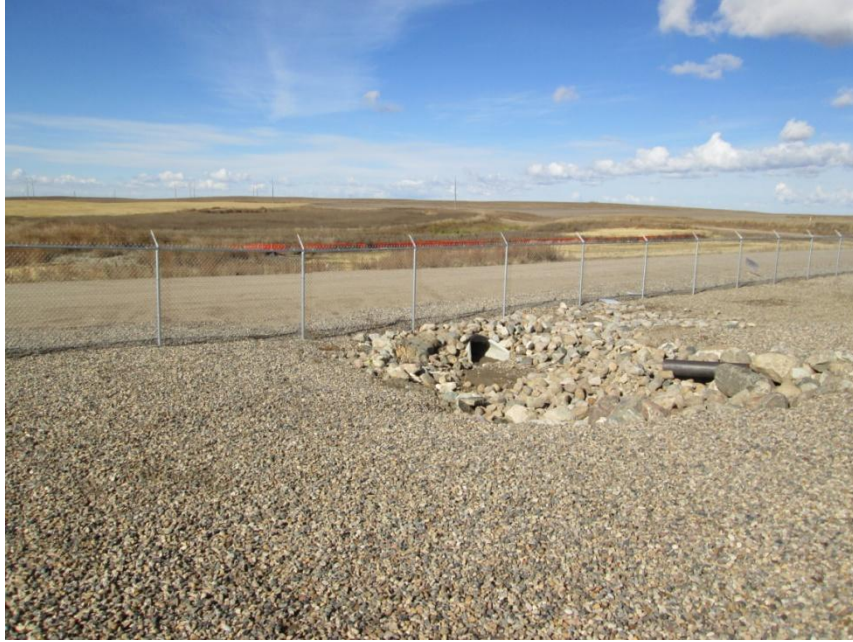
Photo 5. Direction: Northwest. Sediment fence placed near a wetland. Note culverts and rip-rap installed to promote natural drainage and prevent erosion.
