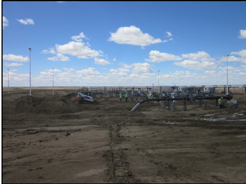
Photo 3. Direction: West. Pipeline tie-in area to the north of the two tanks. At time of visit trenches were being backfilled and electricians were finishing up work. After that, they would be putting clay lining in the area and testing for compaction. In foreground is header to East Fork (pipeline associated with the pump station).
