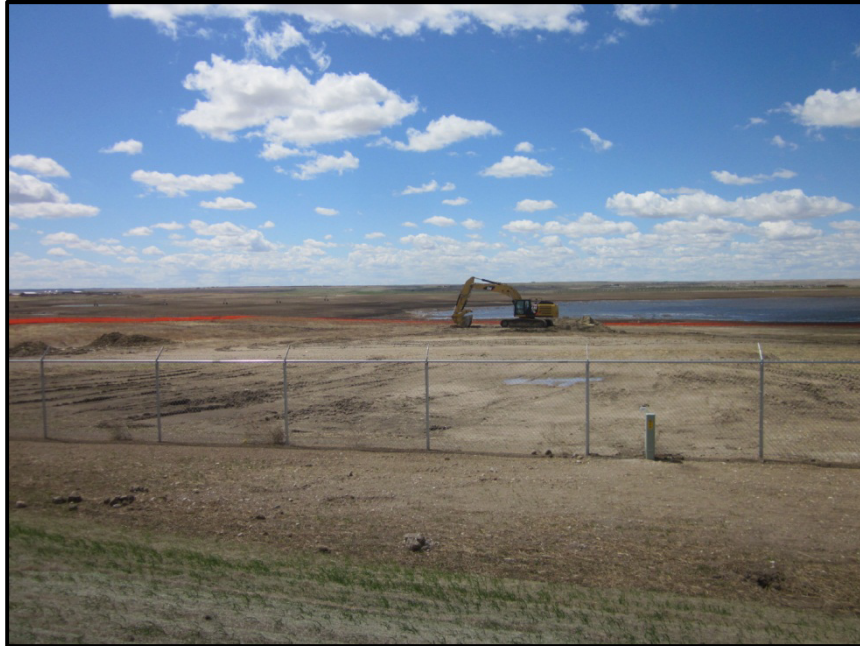
Photo 5. Direction: West. Off west side of pumping station where hydrostatic test waters had been released during pipeline testing. There was still some cleaning up to be done. A silt fence was visible in the distance.
