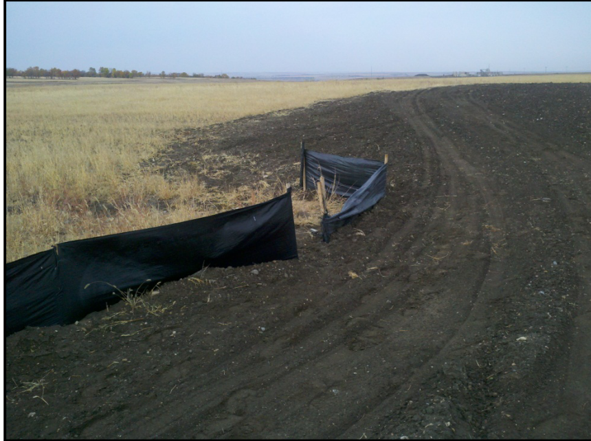
Photo 21. Dry upland field drain with erosion control silt fence in place. The fence is in need of minor repair.
