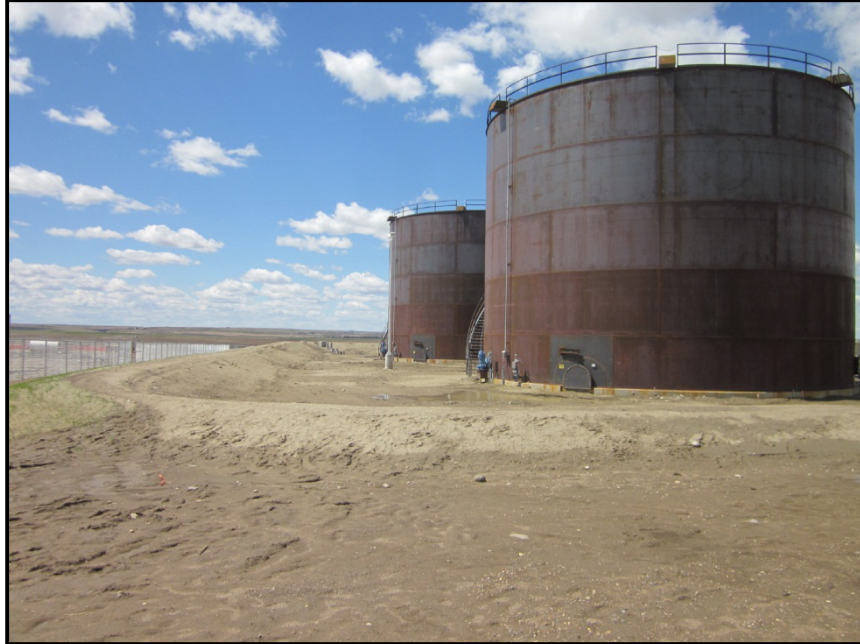
Photo 1. Direction: West. South side of tanks at Little Muddy Pump Station showing spill-containment berm still being put in at the time of field visit. Tanks were to be painted summer 2013. Tanks are 30,000 bbl (oil barrel) capacity; only one will be used at first; the other will be reserved for future use.
