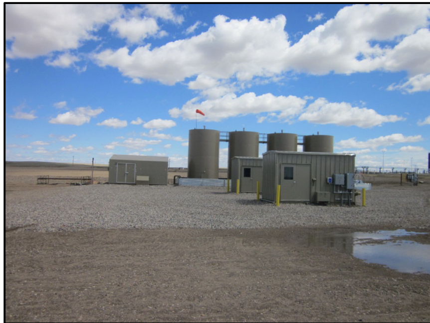
Photo 12. Direction: East. Photo shows one of the leased “LACT” lots. Eight of these lots were built north of the pump station for use by companies to lease and move their oil in Enbridge’s pipelines. Each lot has a hook-up with transfer units and meters which measure the oil.
