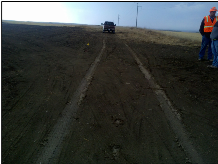
Photo 20. Direction: South. Intersection of pipeline with section line road. Road had been open cut. Everything had been repaired and was in good condition.
