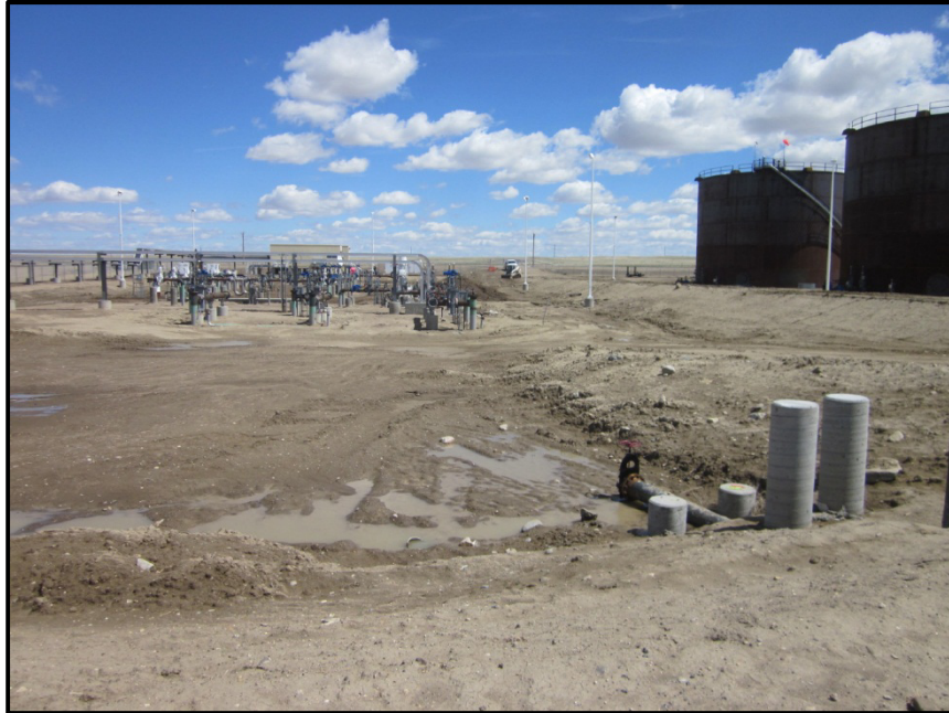
Photo 7. Direction: East. View across site from west to east. Drain valves in foreground release rain water collected within containment berm, which are closed except when drainage is needed.
