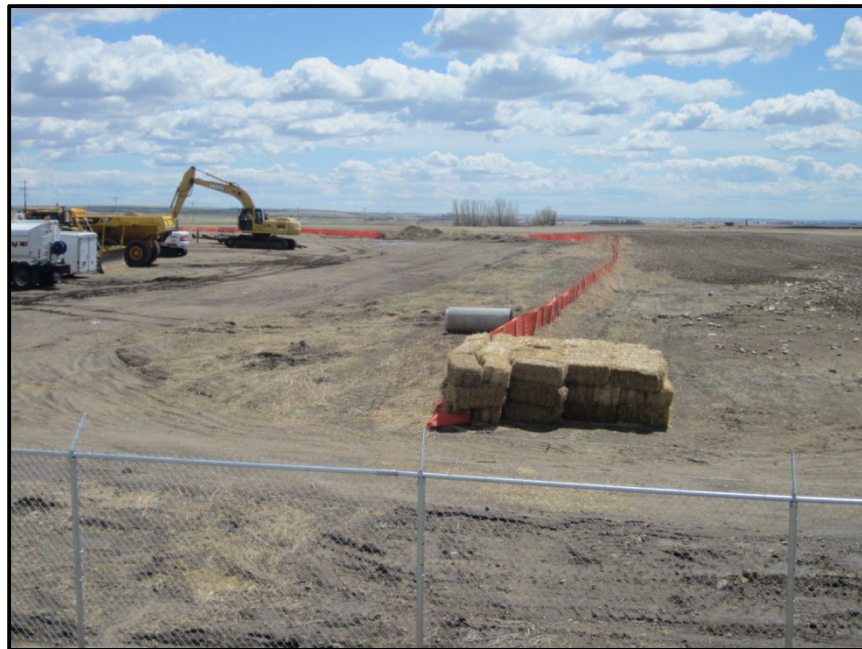
Photo 10. Direction: South. Area to south of pumping station used as a staging and lay down. Bales and silt fence used for erosion control and other various equipment are shown.
