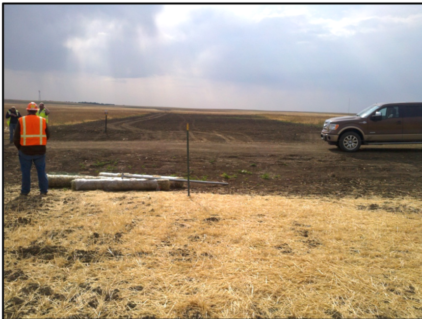
Photo 24. Direction: South. An open cut crossing of a section line road. The road, adjacent ditches and fields, and fences had been repaired properly. No problems were noted.
