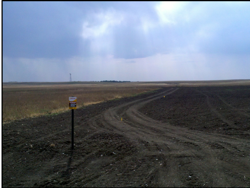
Photo 25. Direction: South. Pipeline was installed across fields and topsoil was replaced to necessary standards.
