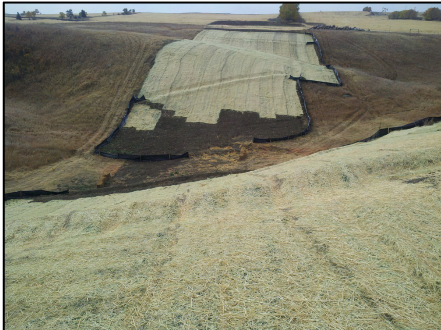
Photo 22. Direction: South. Pipeline route crossed several steep hills with dry drainages at base. In these instances, erosion control blankets were used, the hills were double seeded with local native seed using local NRCS guidelines. Extra straw mulch was used as well as a cover crop of winter wheat. On the distant hill the ROW was reduced to miss the row of trees to the south.
