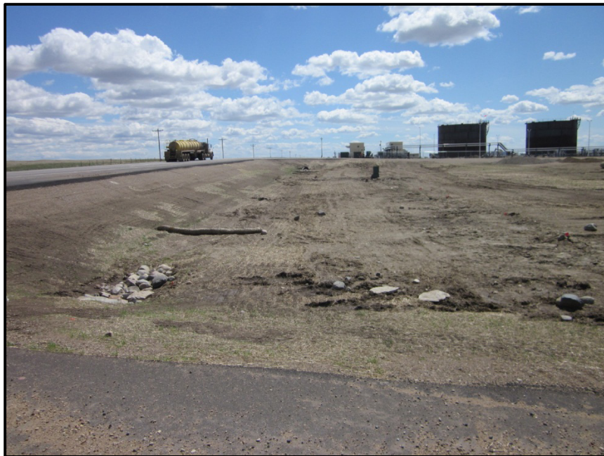
Photo 16. Direction: South. As part of the project Enbridge paved the road leading up to the pump station (133 rd Ave NW). Ditches were reclaimed with erosion control and drainage in place with everything in good condition. A turning lane was added at the approach to the LACT lots to accommodate truck traffic.
