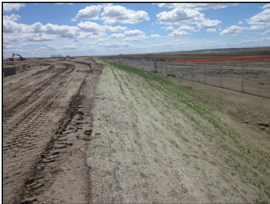
Photo 6. Direction: South. West side of berm around tanks. Grasses had been seeded into erosion control blanket and were coming up well.
