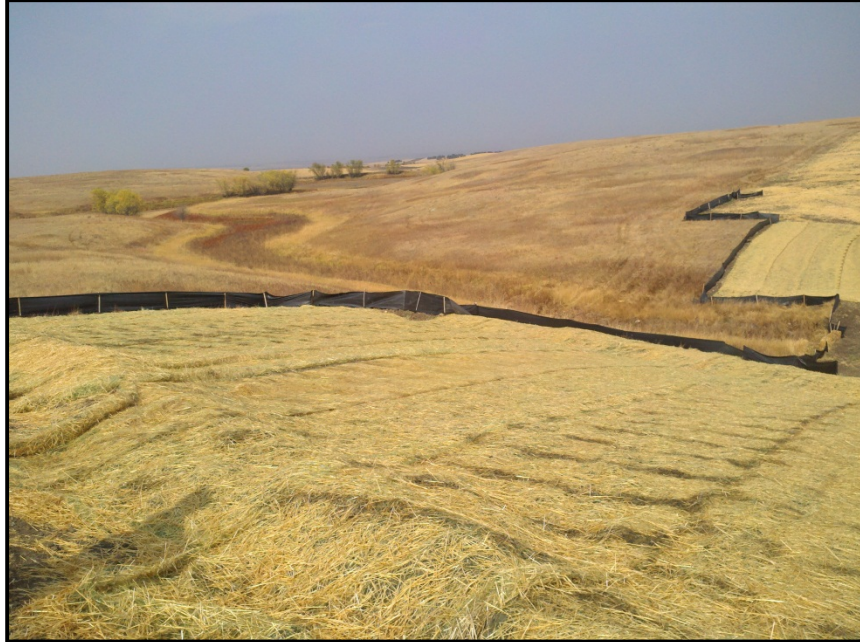
Photo 23. Direction: Northwest. Another steep hill crossing, this one with a wetland drainage at its base. The ROW width had been reduced, but open cut through the wetland. Proper erosion and sediment control and seeding had been done and was effective. Note the water bar in the foreground.
