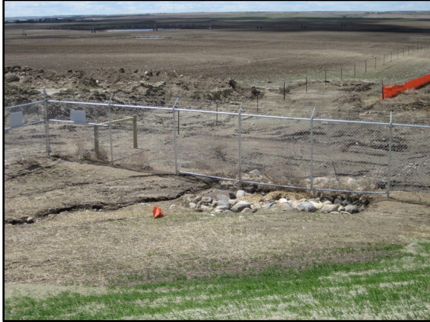
Photo 9. Direction: Southwest. Rip-rap on outside of berm showing where water will exit site when the drain valves are used.
