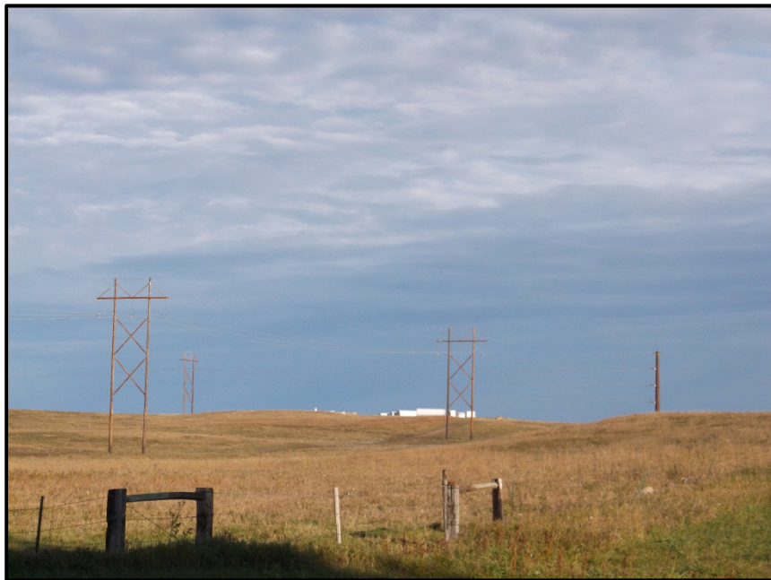
Photo 6. Direction: West. View of a single steel pole structure that changes direction of transmission line to the west.
