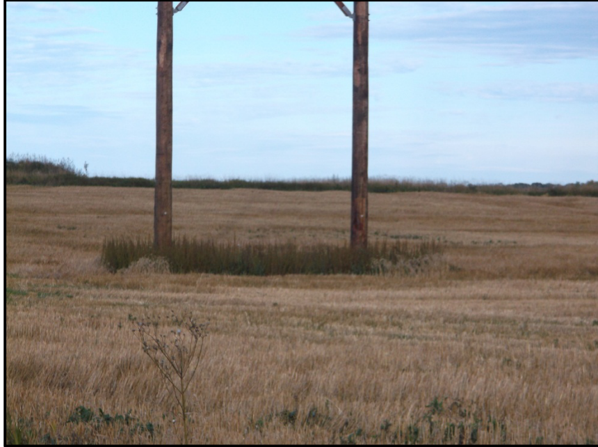
Photo 3. Direction: Northwest. View of base of transmission H-frame structure where reclamation is complete and re-vegetation has occurred.
