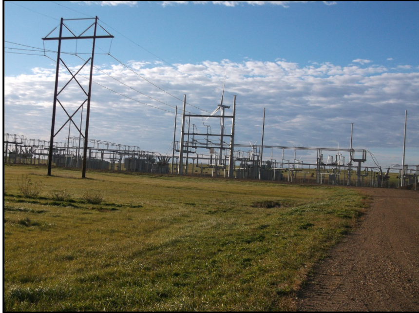
Photo 1. Direction: South/Southeast. View of the transmission line (H-frame structures) on the east end of the route at the Bison substation.
