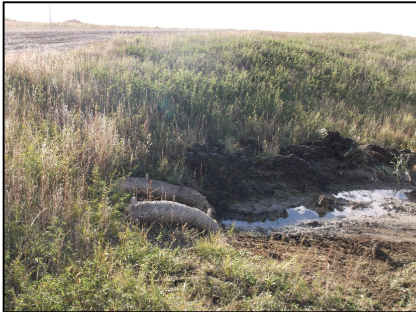
Photo 8. Direction: South/Southwest. View of stormwater straw waddles being utilized to prevent sediment from leaving construction area.
