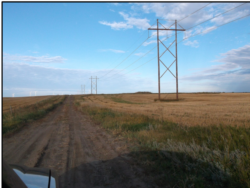
Photo 2. Direction: West. View of the transmission line with bird diverters installed on the transmission line around the wetland. Section line road is also visible.
