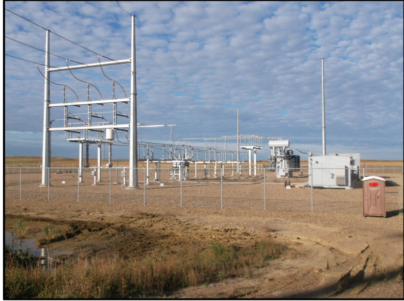
Photo 7. Direction: Southwest. View of the Tri-County substation and wetland that experienced no construction-related disturbance.
