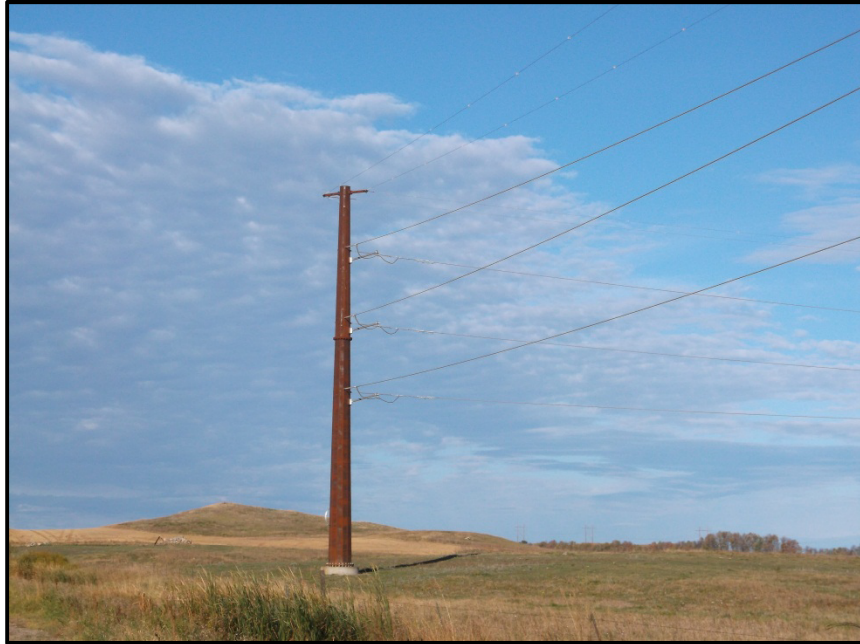
Photo 5. Direction: Northwest. View of a single steel pole structure that changes direction of the transmission line to the north.
