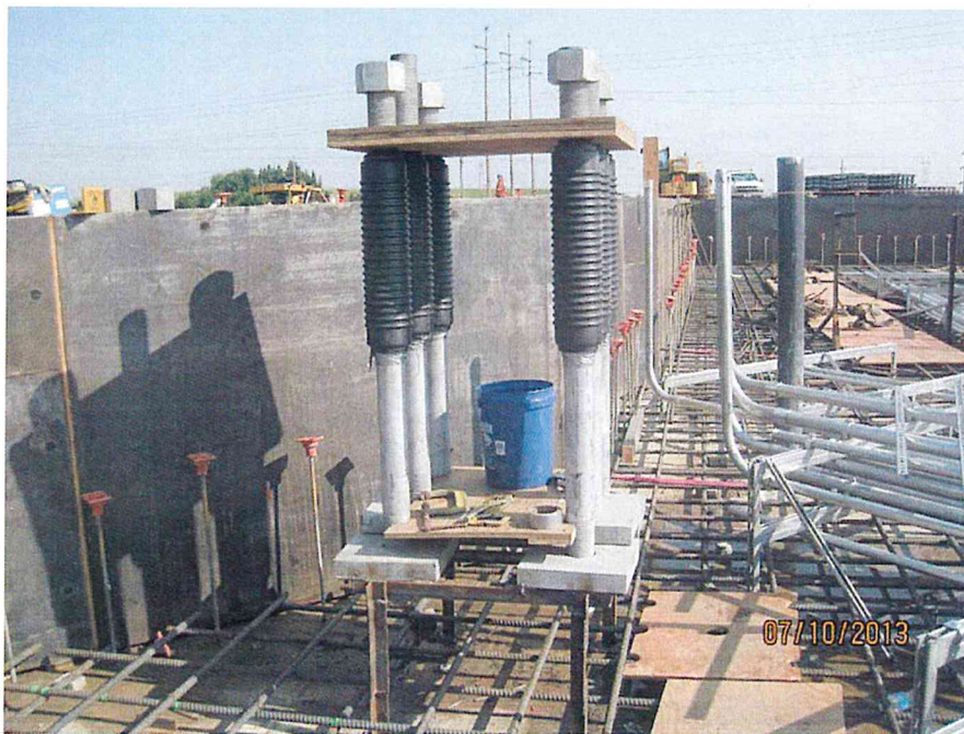
Inlet air plates and bolts in Combustion turbine (looking N)
