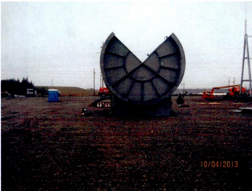
Exhaust stack assembly (looking N)
