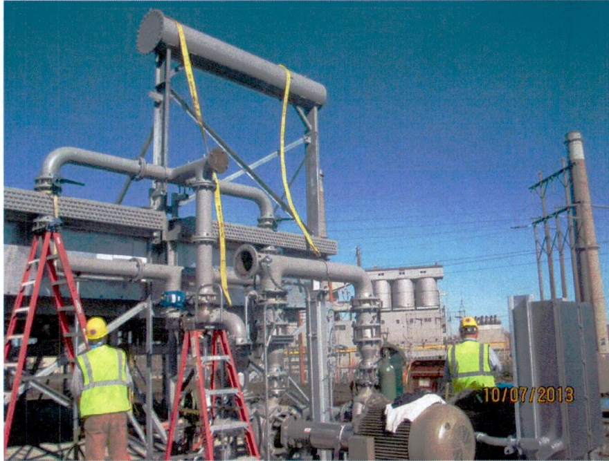
Closed cooling water piping and motor installation (looking NE)
