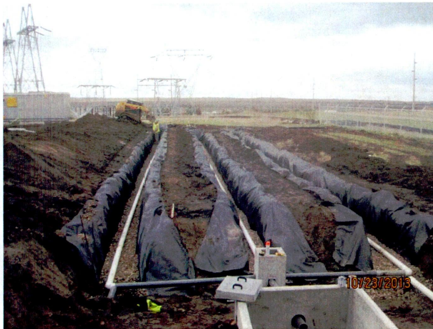
On site wastewater treatment system (looking E)
