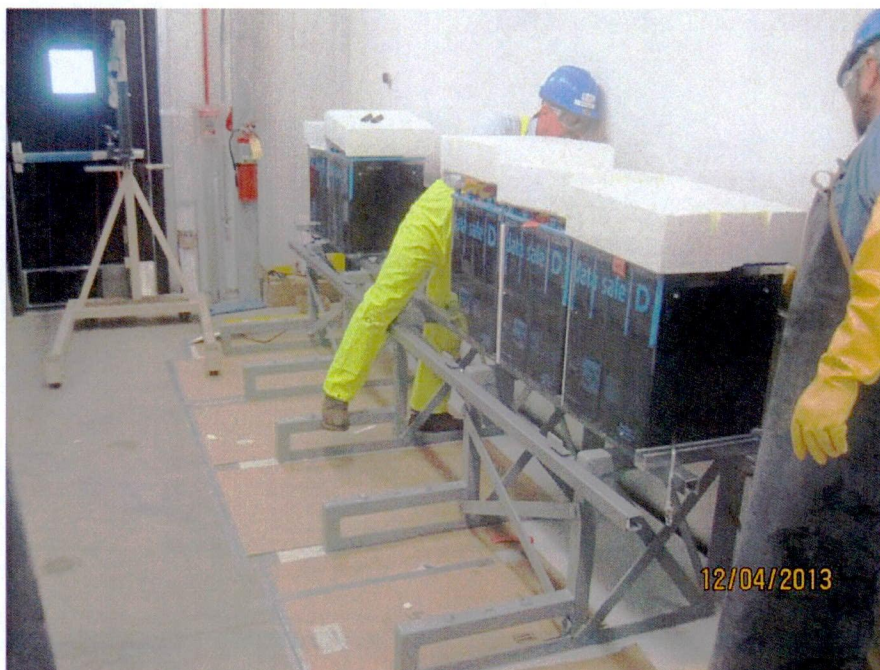
Service Building battery installation (looking W)
