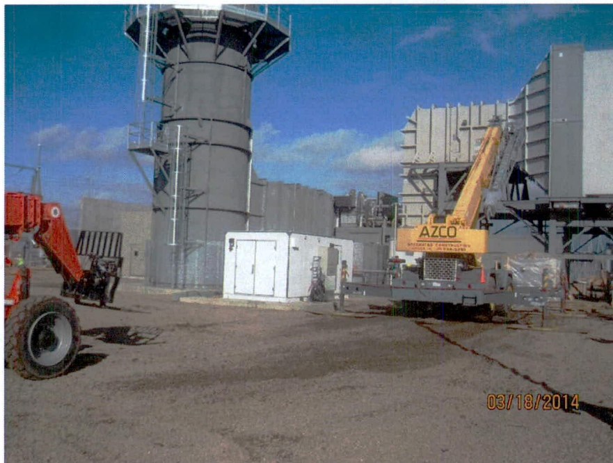
CEMS enclosure set (looking NE)
