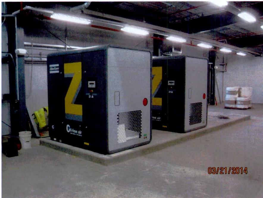
Service Building air compressor installation (looking SW)
