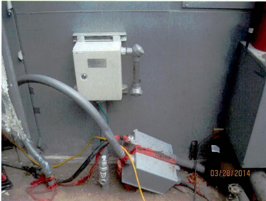
Junction box terminations (looking E)
