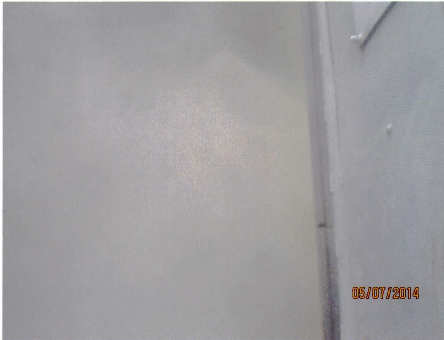
Accessory enclosure fire mist testing (looking E)
