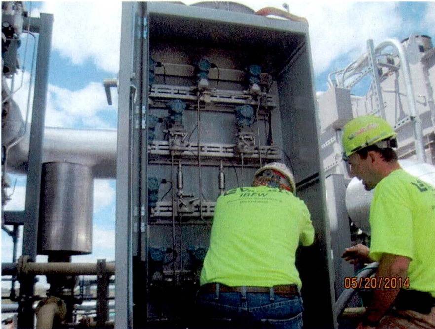
Instrument heated box installation (looking W)
