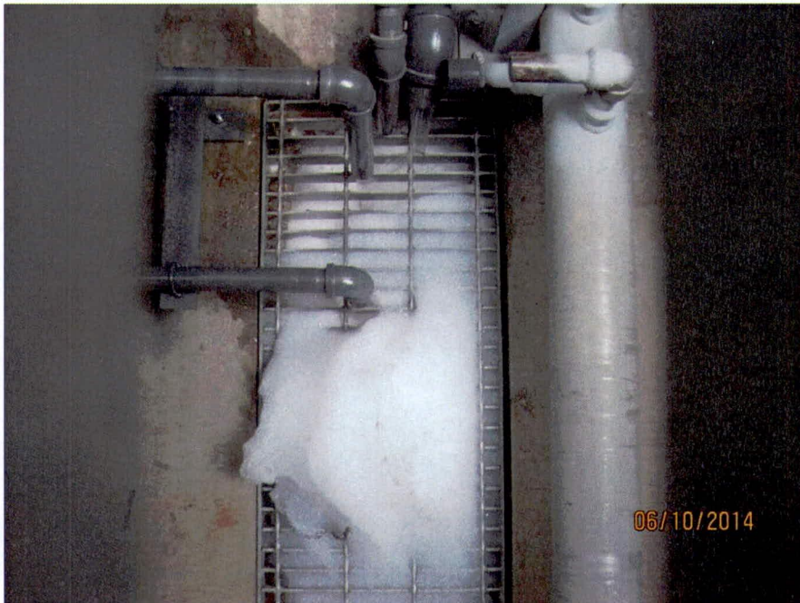
Turbine water wash discharge (looking N)
