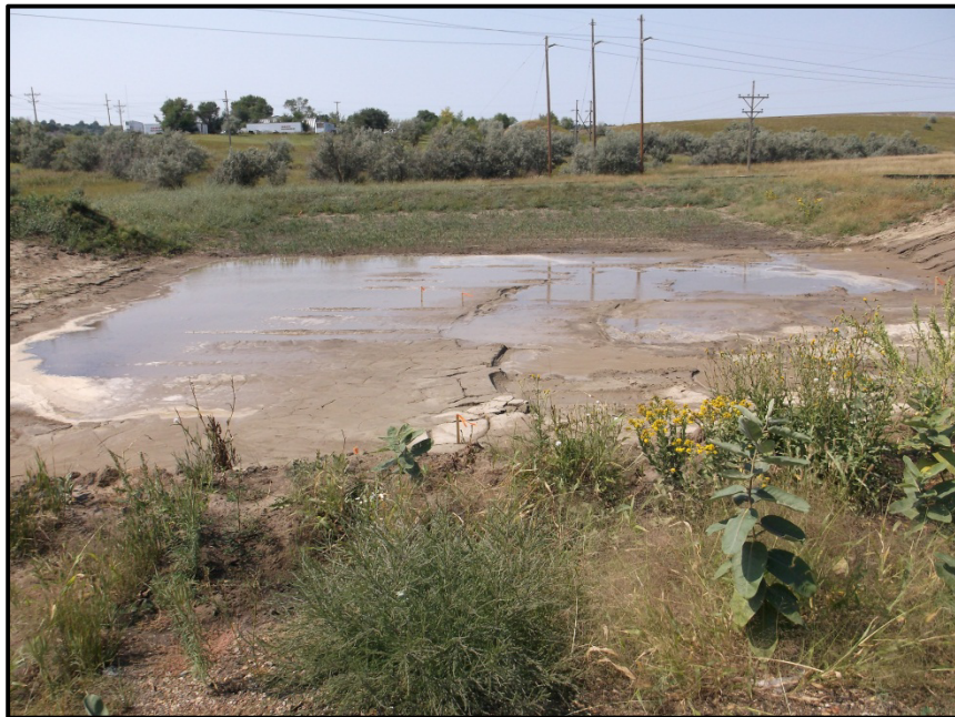
Photo 6. Direction: West. View of future stormwater pond. At the time of this photo it was under construction.
