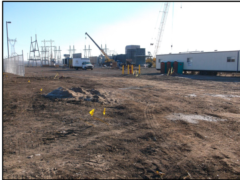
Photo 16. Direction: South/Southeast. Overall view of entire project site, during construction of the 88 MW turbine. Note that the site and working area is clear of debris and trash.
