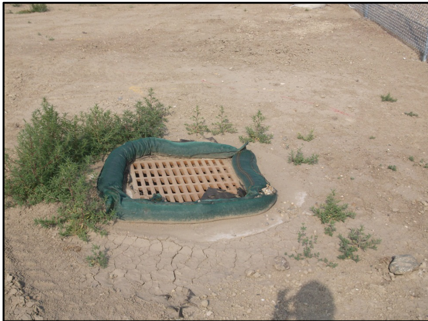
Photo 2. Direction: West. Additional view of stormwater inlet protection on the project site.
