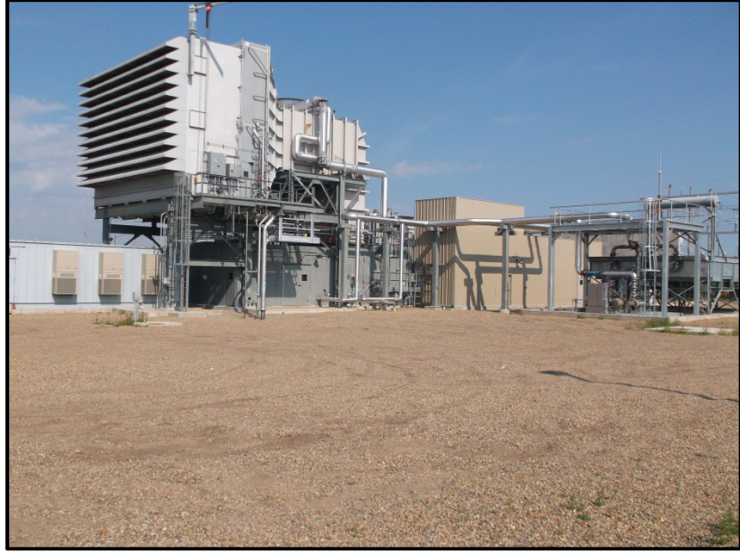
Photo 13. Direction: Northwest. View of the MDU 88 MW combustion turbine and graded project area.
