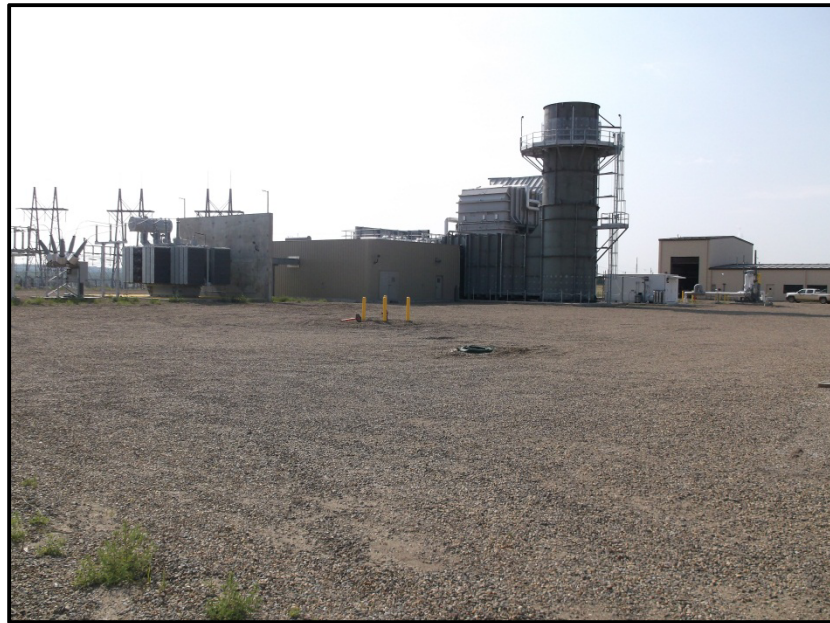
Photo 8. Direction: Northwest. View of stormwater inlet protection (in foreground) and MDU 88 MW turbine. Note the grading and surface gravel of the project site.
