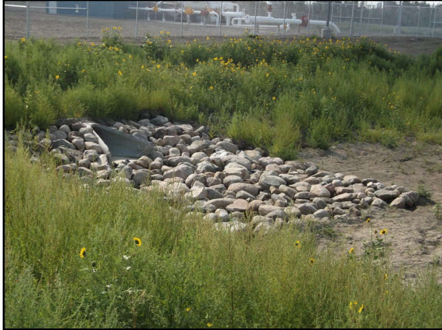
Photo 5. Direction: Southwest. View of stormwater drainage outlet surrounded by riprap and reclamation growth.
