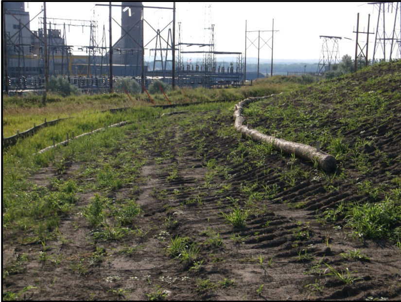
Photo 14. Direction: East. View of stormwater straw waddles being utilized to prevent sediment from leaving construction area.
