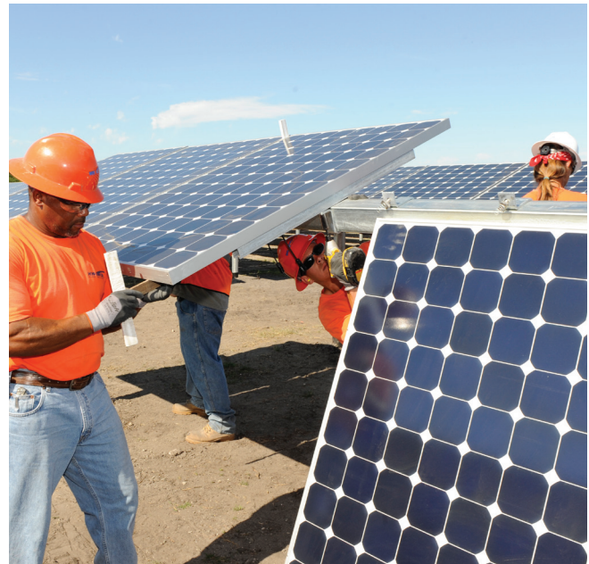
FPL's Space Coast Next Generation Solar Energy Center began delivering clean, emissions-free solar power to Floridians in 2010
