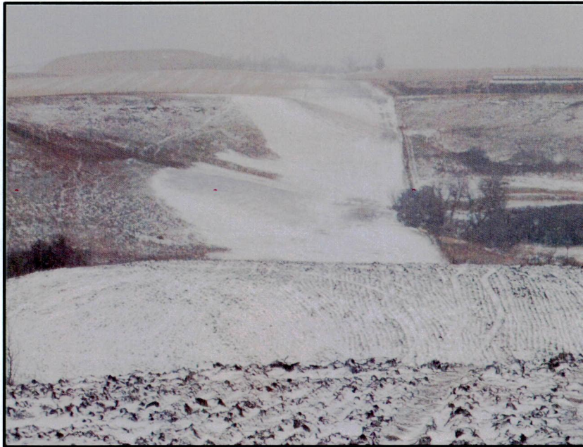
Photo 5. Direction: North (GPS Point #58). Pipeline route passes through sandy hills, requiring large cut sections. Topsoil was imported and placed on top of disturbed area to help control erosion.
