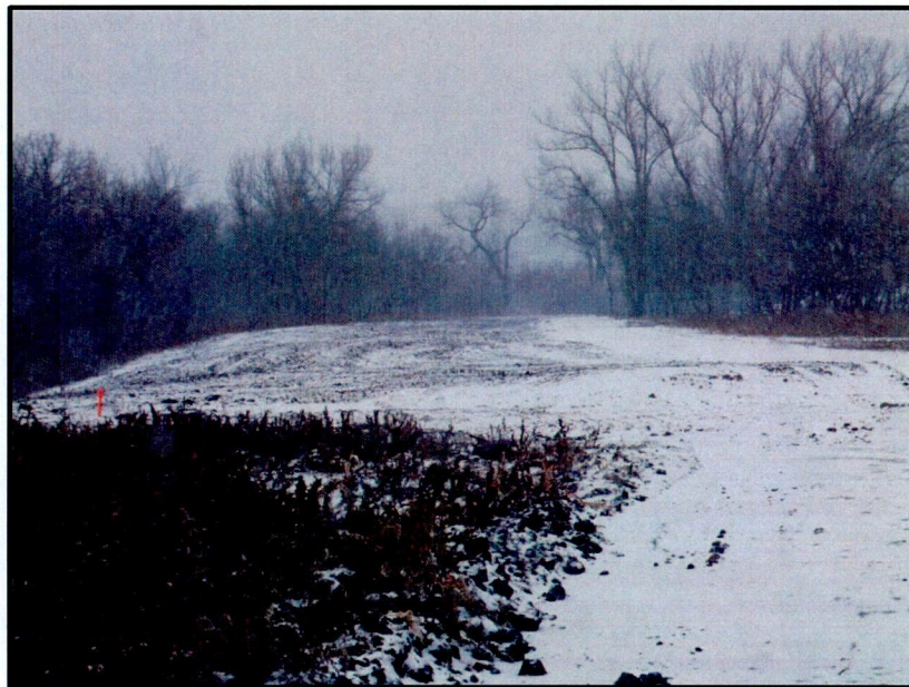
Photo 4. Direction: North (GPS Point #49). Pipeline passes through wooded area; some trees removed.
