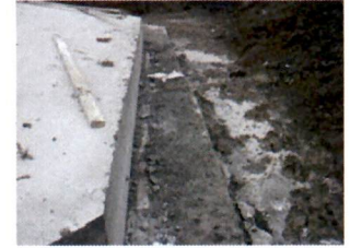
Mud Slab and Turbine Foundation 300 Cubic Yards of Concrete for the Slab, Foundation, and Pier
