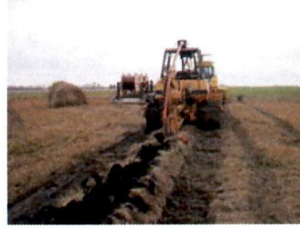
Electrical Collector 17,300 Linear Feet from Campus to Turbine Site
