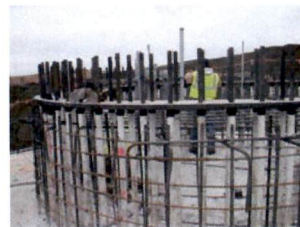
Pier Reinforcing and Tower Anchor Assembly 140 Anchor Bolts in PVC Sleeves from Embedment Plate
