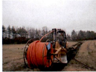
Primary Conductors and Conduit for Fiber Optics
