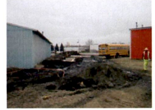
Electrical Interconnection Location - Step Up Transformer, Grounding Transformer, Switchgear and Hut
