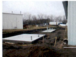
Electrical Interconnect Location Ready for Transformers, Switchgear, and Communications Hut
