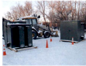
Step Up and Step Down Transformers Await Installation
