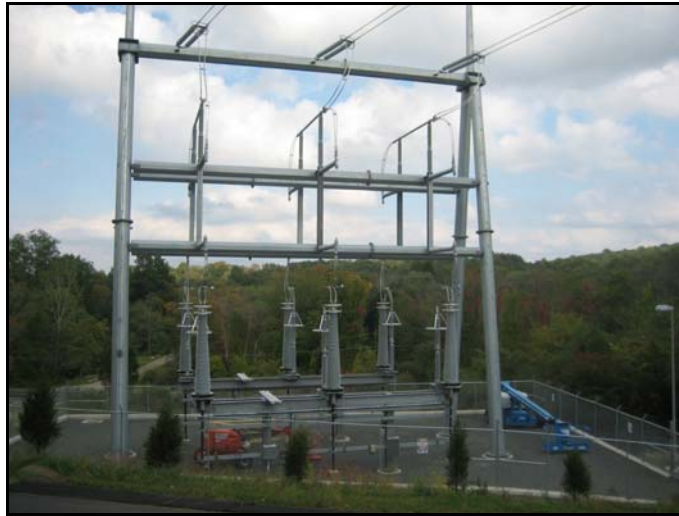
Figure 7 Small Transition Station
