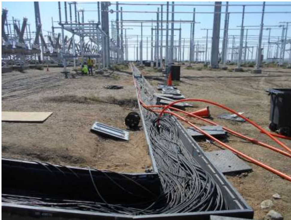
Photo 2 – Electrical wiring enclosure. Fiber optic cabling located in orange conduit.
