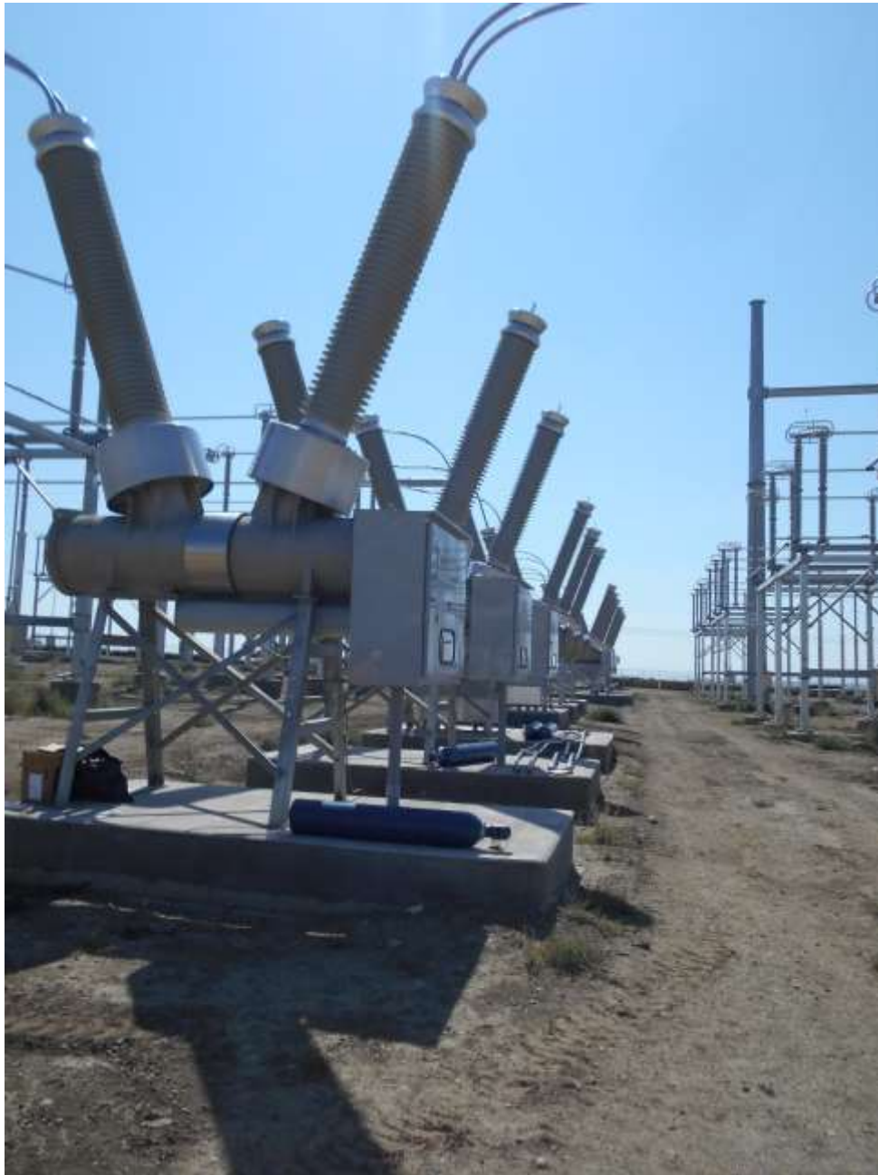
Picture 5 – Electrical breakers looking south.
