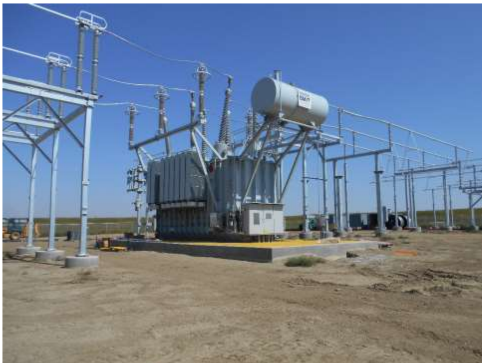
Picture 4 – Electrical transformer looking northeast.
