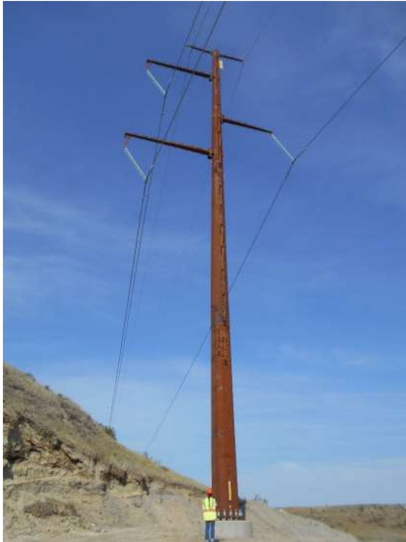
Photo 2 -Typical "Rust" Type of Structure.
