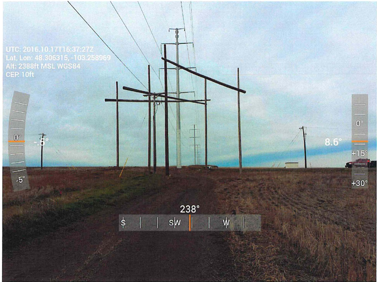
Photo 2 – Transmission Line crossing road with powerline goalposts.
