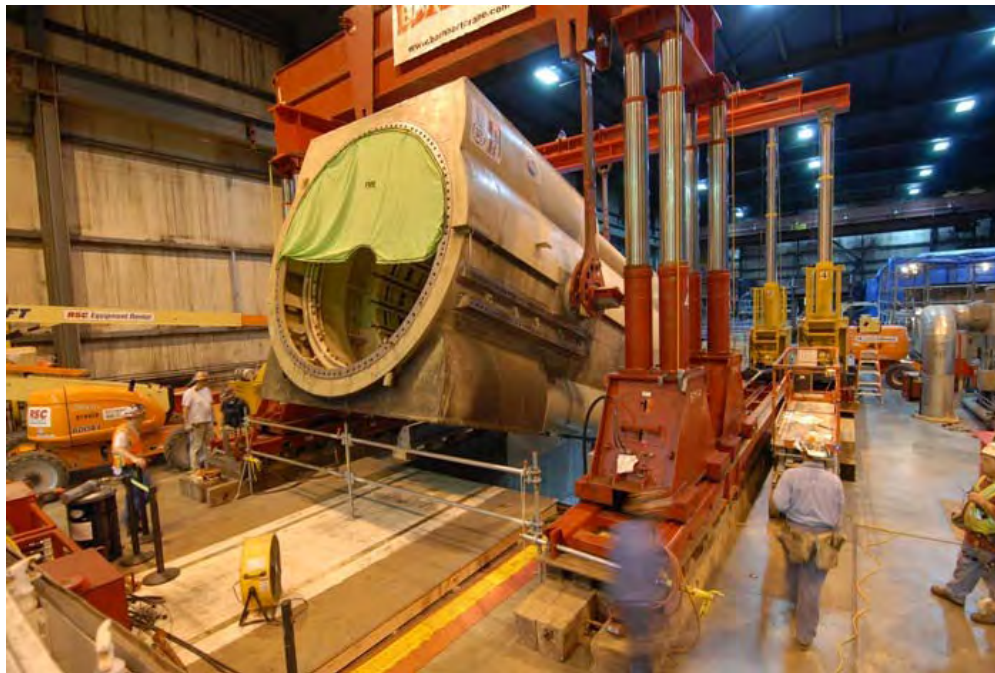
Picture 1: The generator stator being lifted to a vertical position for restacking.
