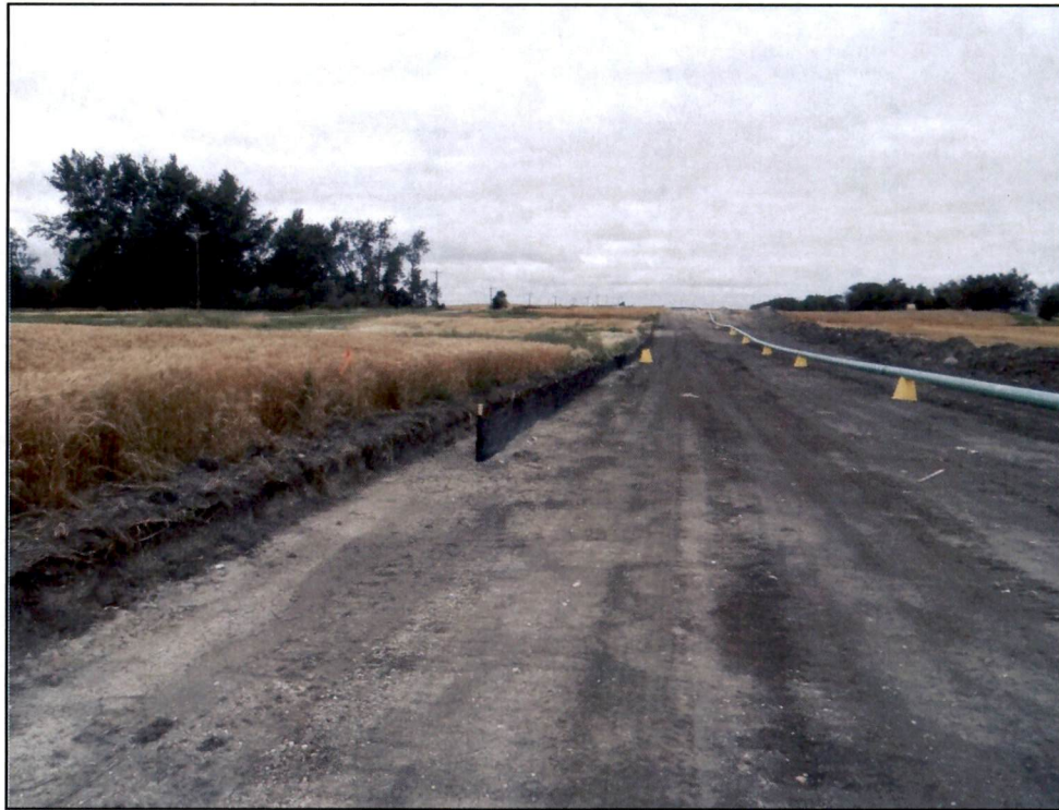
Figure 11. Photo of silt fence placed at edge of the ROW in an area of potential surface water intrusion onto the ROW.
