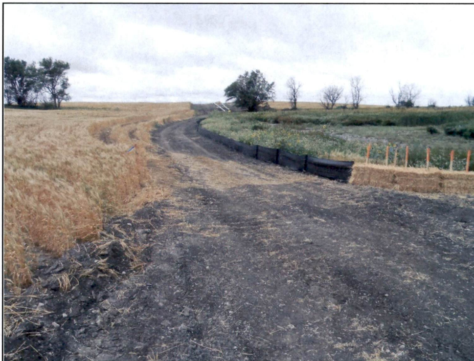
Figure 6. USFWS easement wetland avoided within an agricultural field. The easement wetland will be bored under. A travel corridor is established around wetland and protected by silt fence and straw bales.
