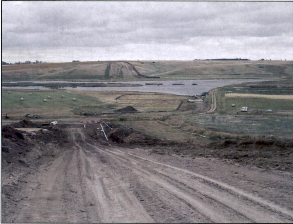
Figure 9. East facing overview photo of Little Knife River planned west side of bore pit work area.
