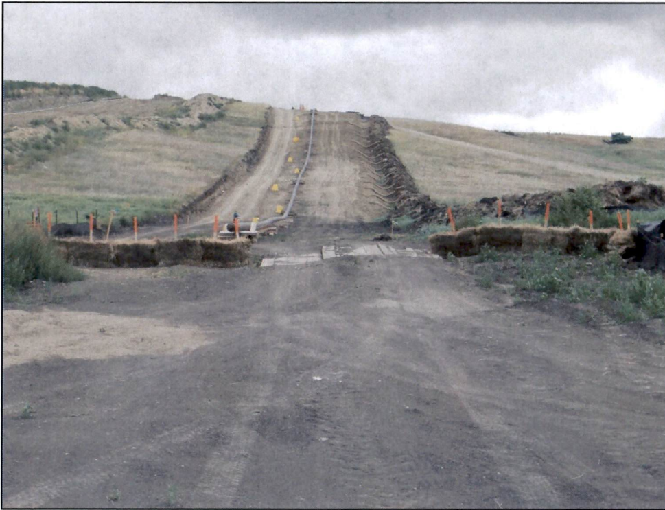
Figure 7. Photo taken facing east along ROW from east side of the Little Knife River. Straw waddles are utilized in slope trenches, slope breakers are placed across ROW where topsoil is removed, straw bales and silt fence are placed across ROW at bottom of slope.
