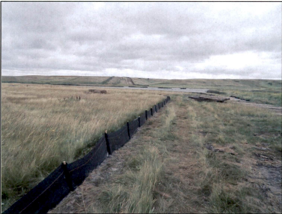
Figure 10. Bore pit work area in flat above water edge with silt fence installed. Wooden mats were in place to allow soil sample truck to drill at planned bore pit location (right).
