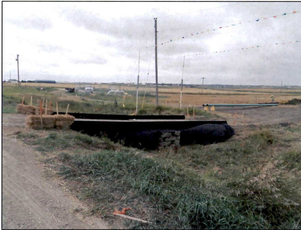
Figure 1. Typical wooden mat bridge at roadway ditch crossing. Additional protection provided by geofabric lining placed under mat and straw bales placed at edges.
