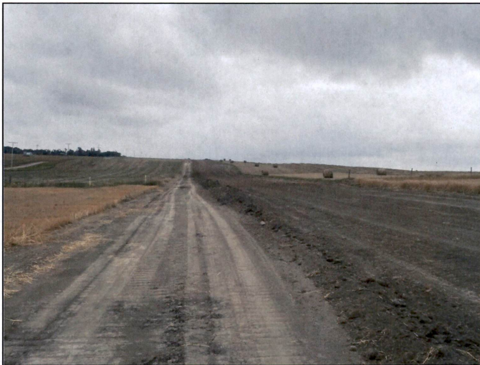
Figure 2. Partially reclaimed ROW. Pipeline installed, trench backfilled and topsoil spread. Topsoil not spread on travel corridor still in use.
