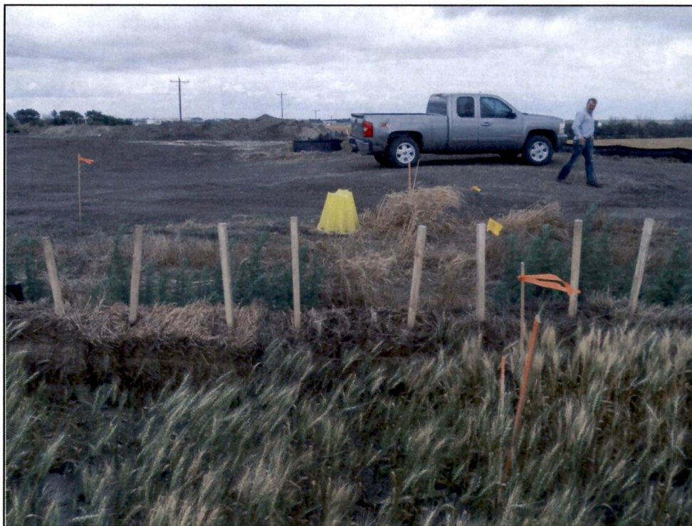
Figure 12. Foreign pipeline marking at ROW crossing. Additional soil placed on top of pipeline crossing per request of pipeline owner.
