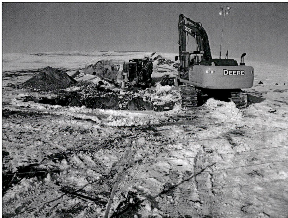
Figure 4. New west side LKR HDD bore pit location. The pit location was moved to avoid wetlands adjacent to the LKR and multiple foreign pipelines.
