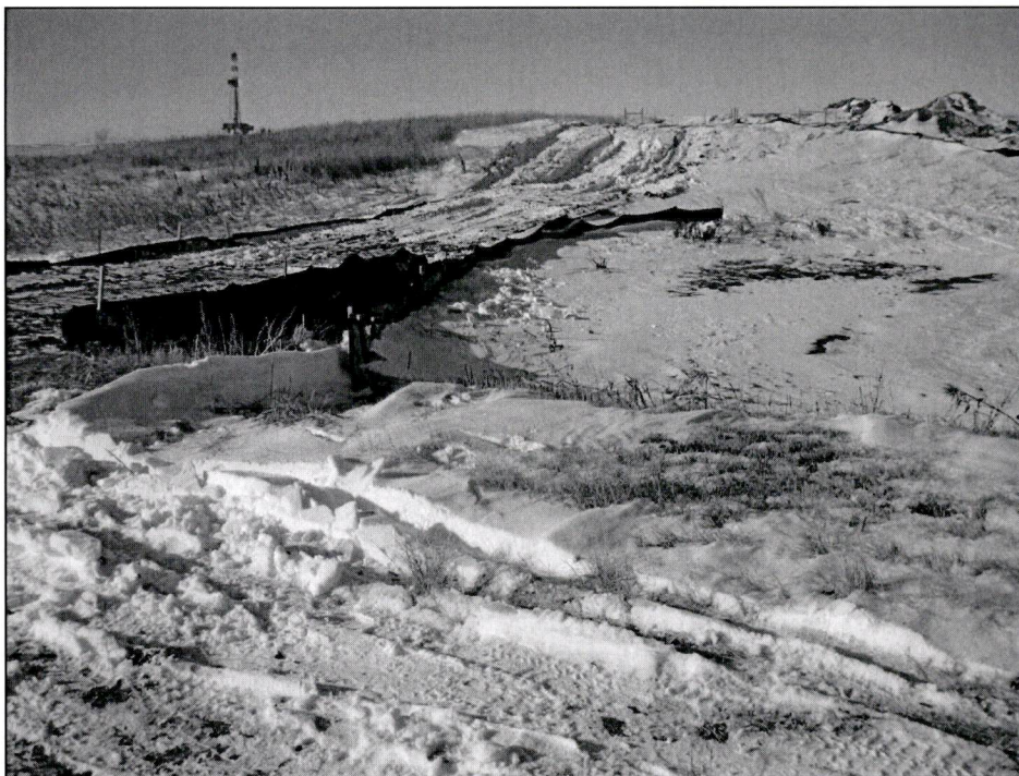
Figure 7. Photo of ECDs utilized to minimize surface impact of wetland while staying within the ROW. Wetland will be crossed utilizing HDD.
