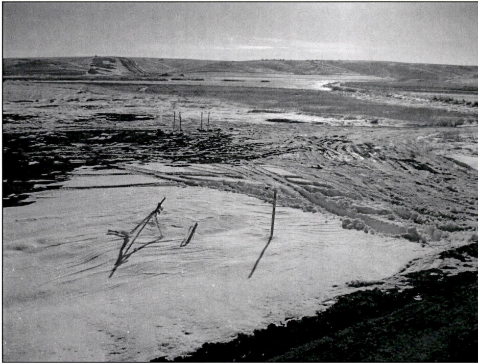
Figure 3. East facing photo of west side LKR prior bore pit work area. Silt fence has been removed and no further surface disturbance has taken place in area.
