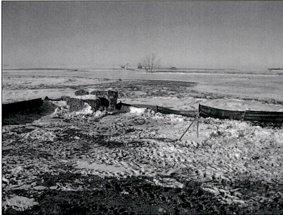
Figure 5. Planned HDD of large wetland complex. Setback was marked and ECD's have been repaired after heavy snowfall.
