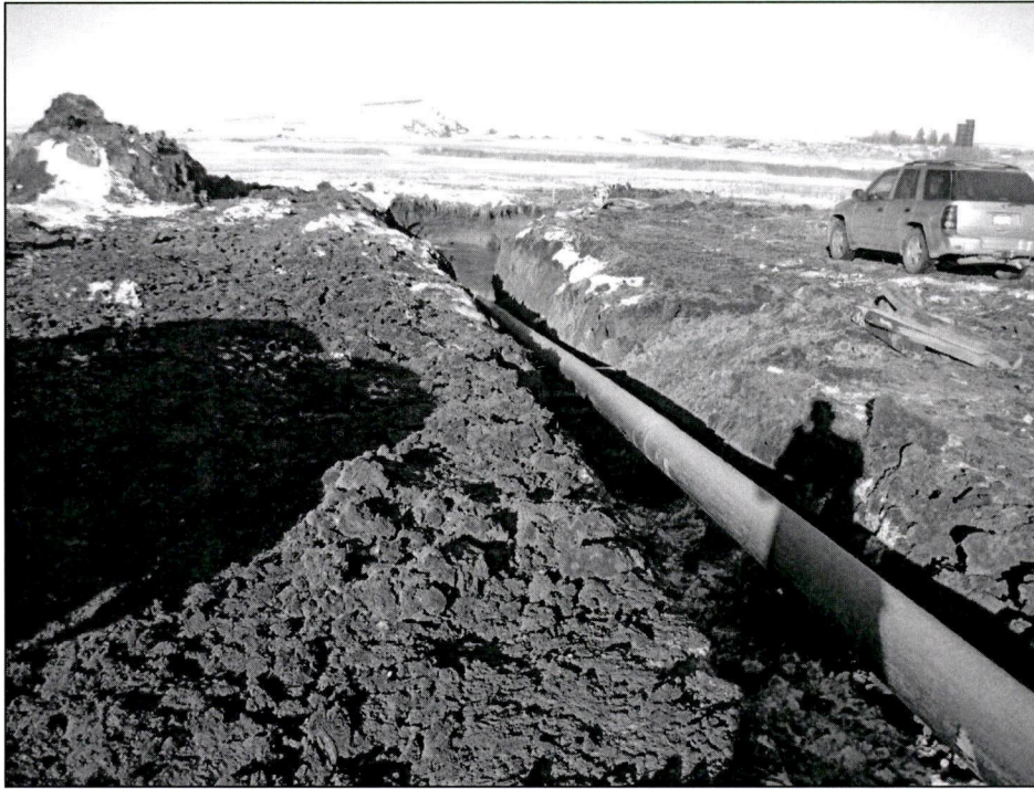
Figure 1. Photo taken looking west along ROW from west side of the Little Knife River (LKR). The HDD bore pit work area was staked and appropriately set back from wetland.
