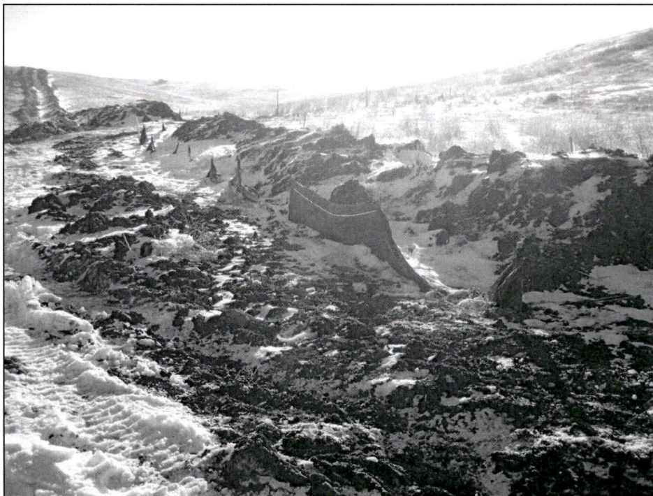
Figure 2. Photo of downed silt fence due to recent snowfall. Silt fences will be temporarily repaired and when ROW reclamation occurs permanent ECD's will be erected.
