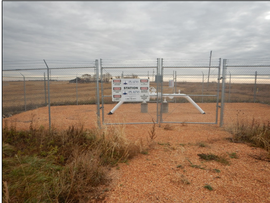
Photo 1. Pipeline above ground valve station. Sites are fenced and gates locked for security and safety.
