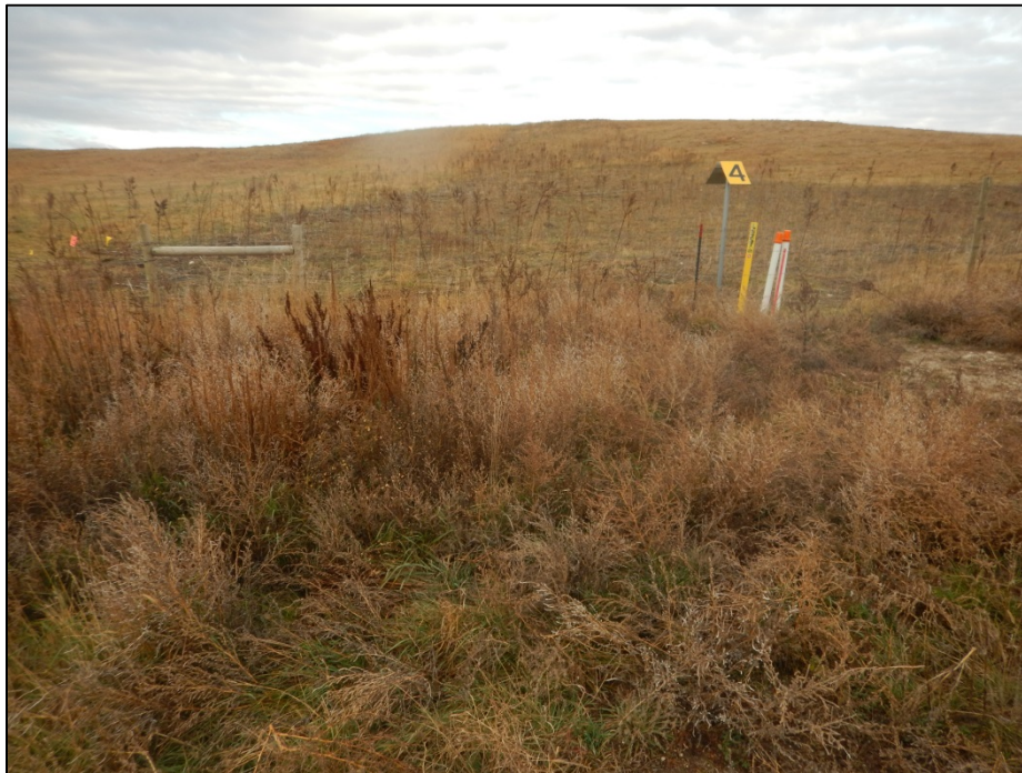
Photo 5. Directional Drill exit hole area under Little Knife River. Rangeland grasses were planted in the summer/fall of 2013 and reestablishment of rangeland appeared to be in satisfactory condition.
