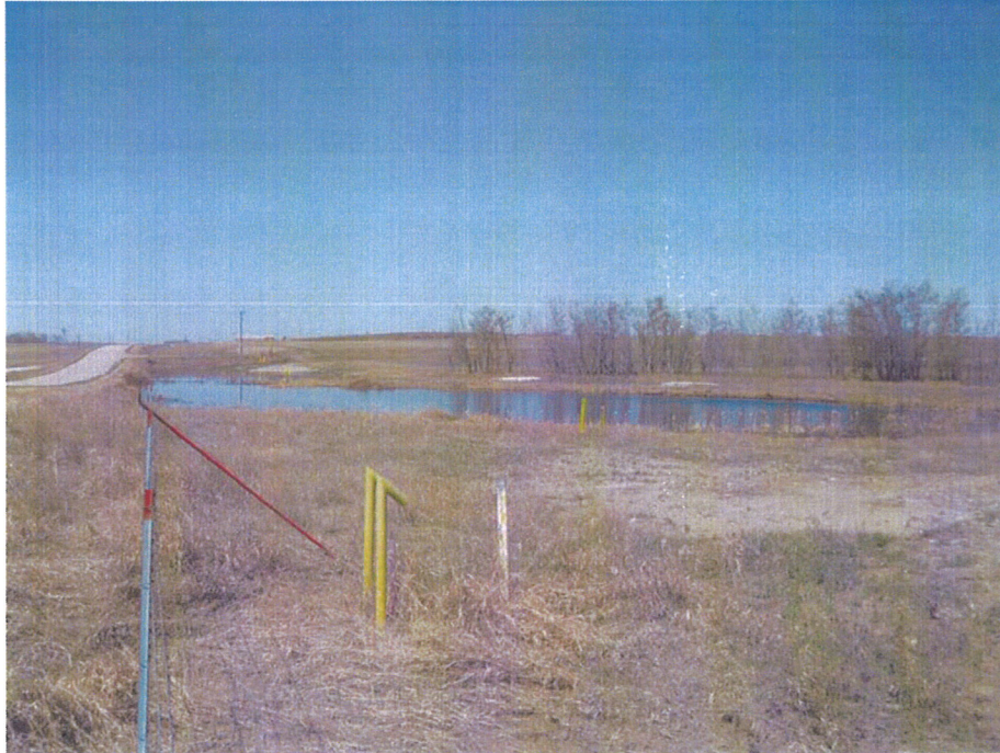
Photo 8 Erosion concern waterways
