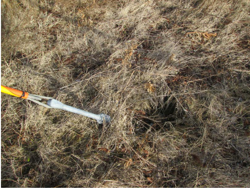
Above: Photo 9 (Structure 452) – Small hole approximately 6 inches deep where guywire anchors from 3-pole structure connect to the ground.
