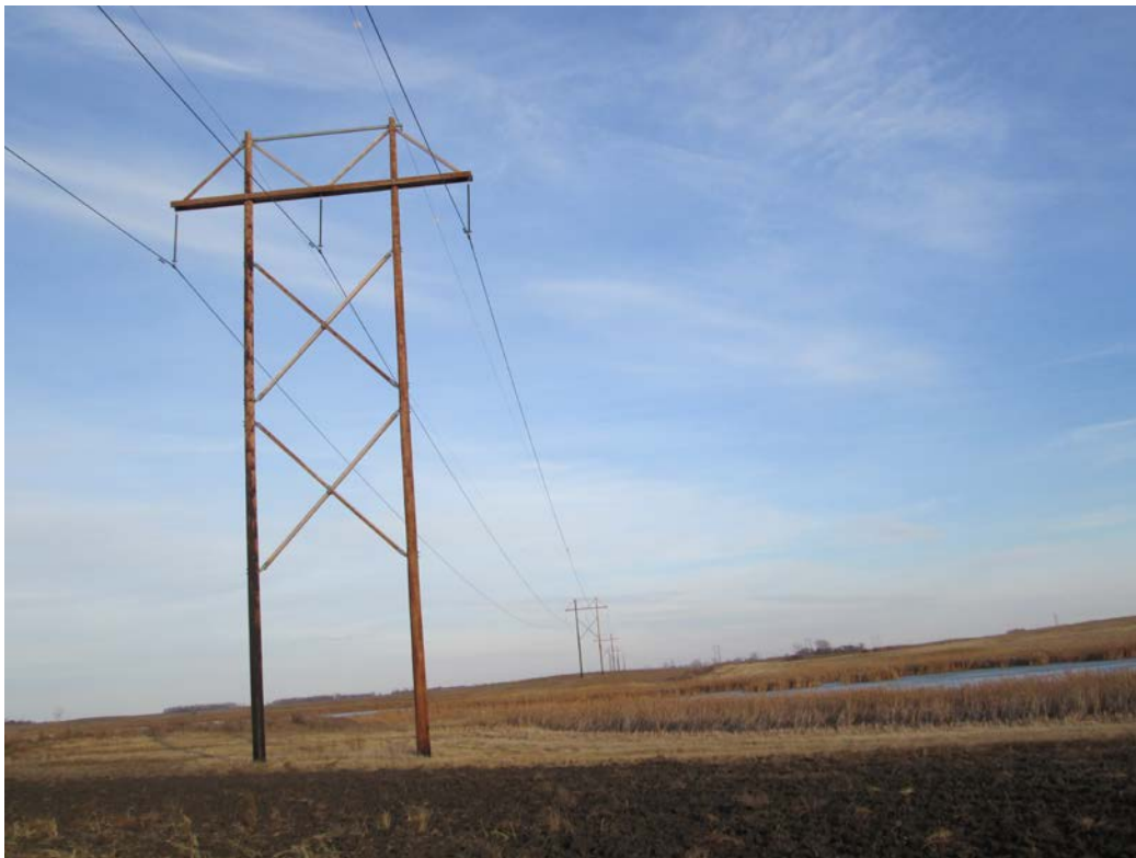
Below: Photo 16 (Structure 561) – Double pole structure next to agriculture field crossing over wetland. Bird diverters along line. Looking northeast.
