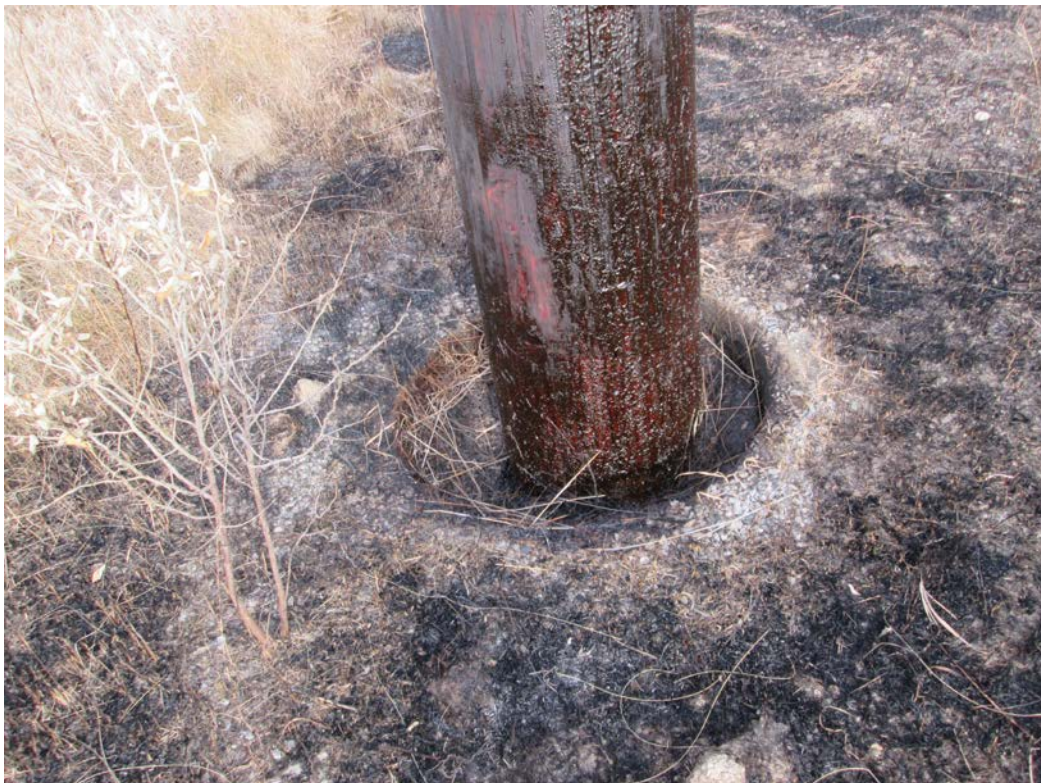
Below: Photo 2 (Structure 459) – Structure's base is below ground level, shows possible settling.
