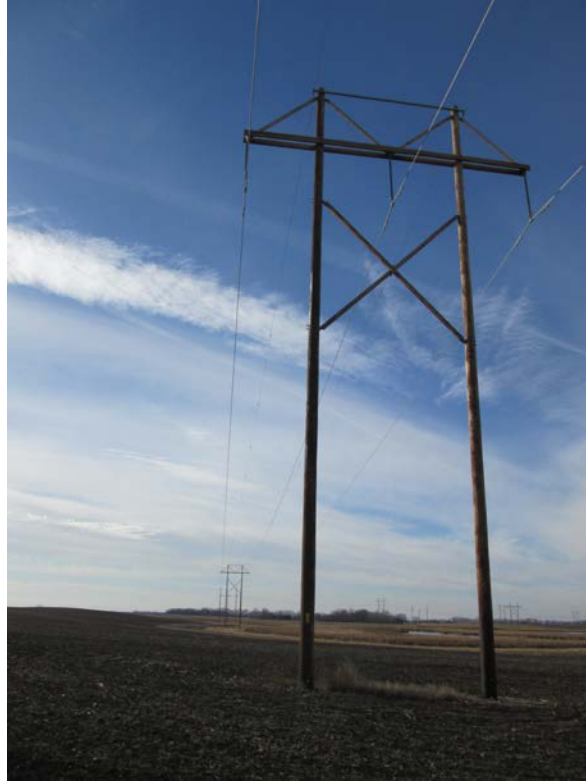
Above: Photo 15 (Structure 450) – Double pole structure along agriculture field and near wetland. Looking southwest.
