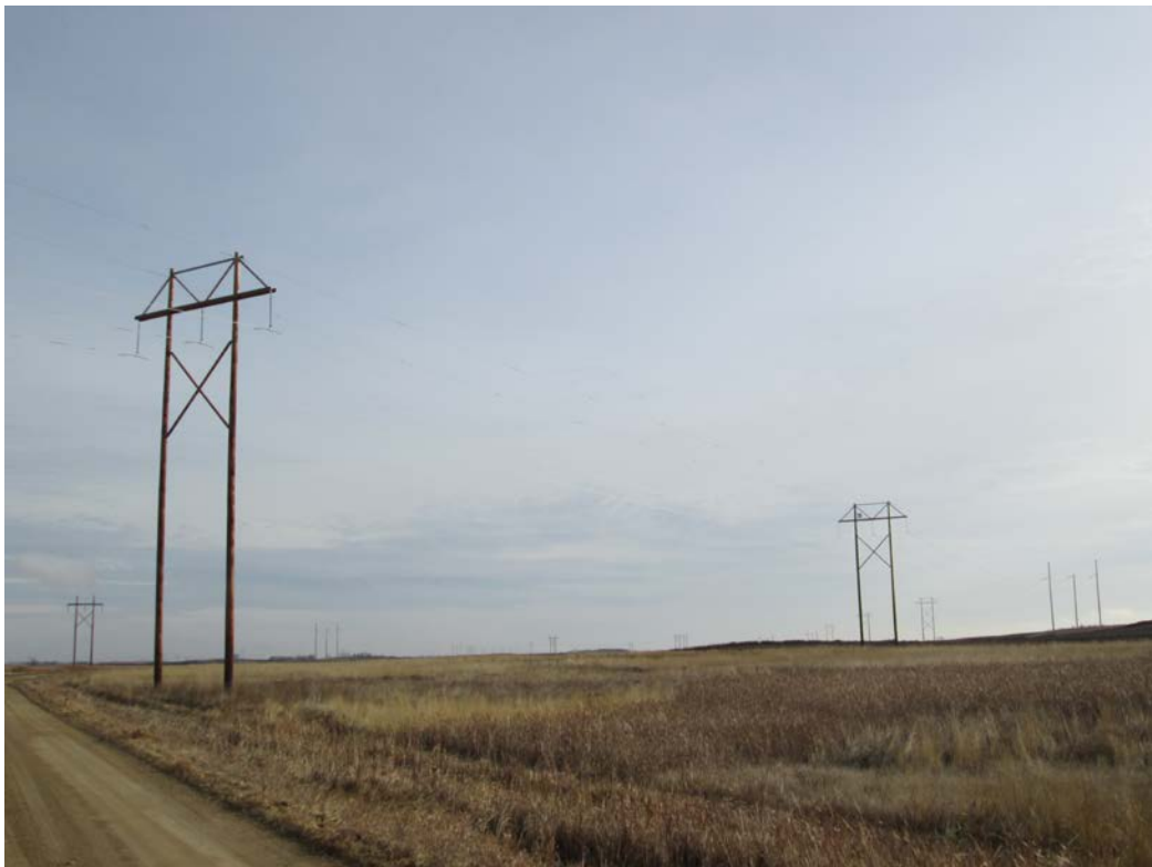
Below: Photo 4 (Structure 458) – Typical double pole structures with H-frame cross arms and braces. Looking east.
