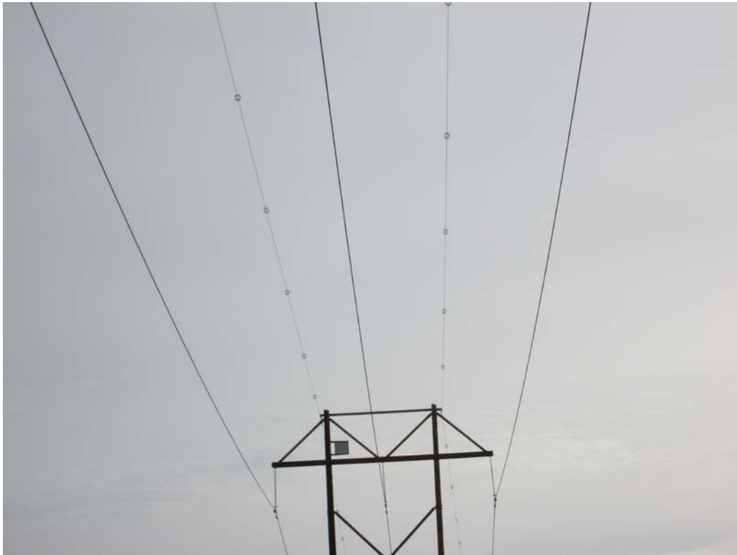
Above: Photo 5 (Structure 457) – Typical double pole structure showing bird diverters along line. Looking southeast.
