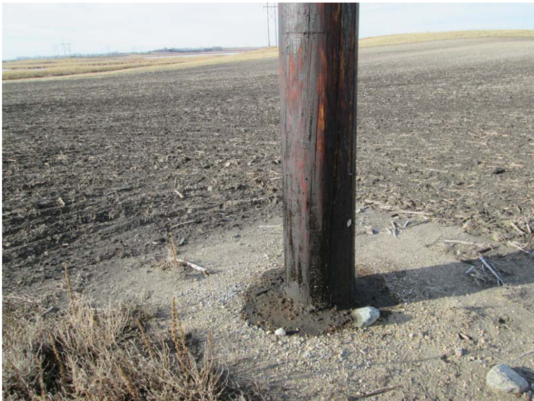
Below: Photo 8 (Structure 450) – Dark stained soil/rocks around the structure. Weeds were observed between the 2 poles of the transmission line structure (only one pole shown).
