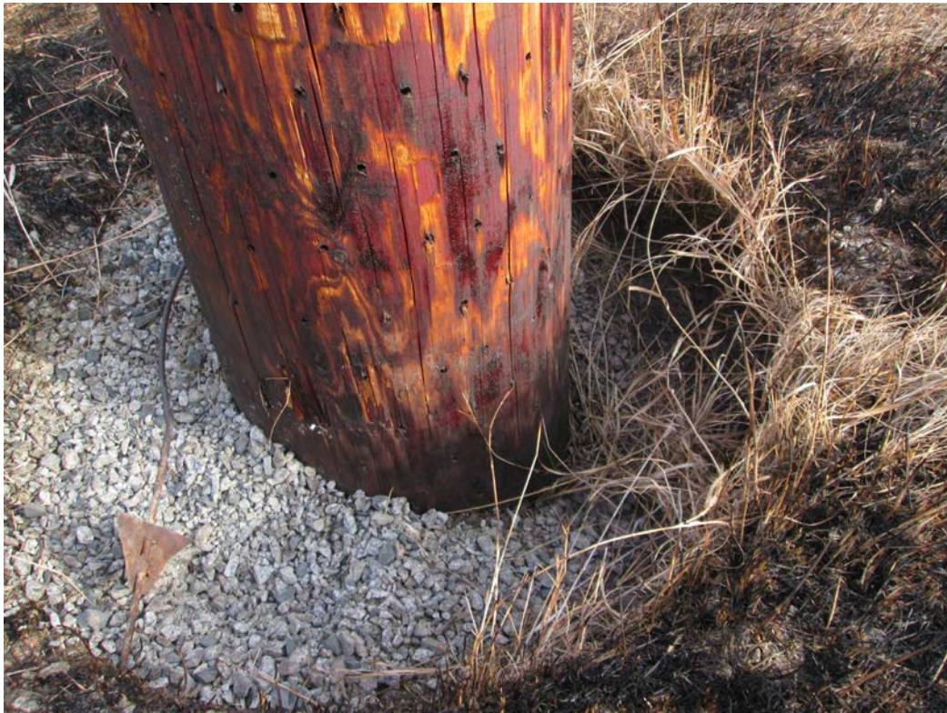
Above: Photo 3 (Structure 459) – Structure's base shows possible settling, as rocks are below ground level, shown on the right side.
