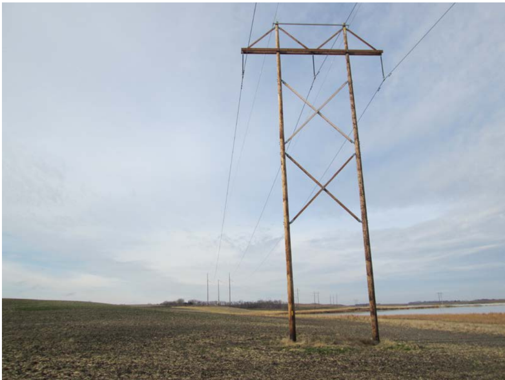
Below: Photo 10 (Structure 455) – Structures going through agriculture field. Weeds and grasses between poles of structure.
