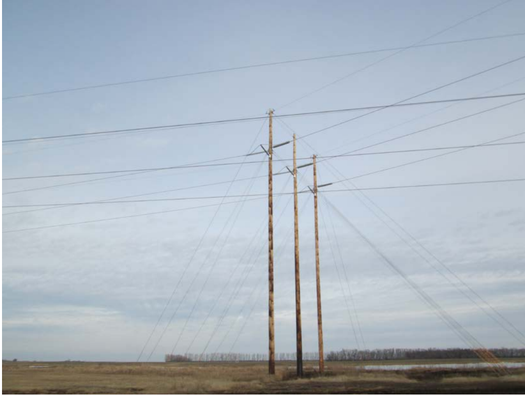
Above: Photo 1 (Structure 459) – Reroute connection to existing transmission line structure at west end of Segment 7 reroute of the Project in Nelson County. Part of the field below had been burned. Looking northwest.
