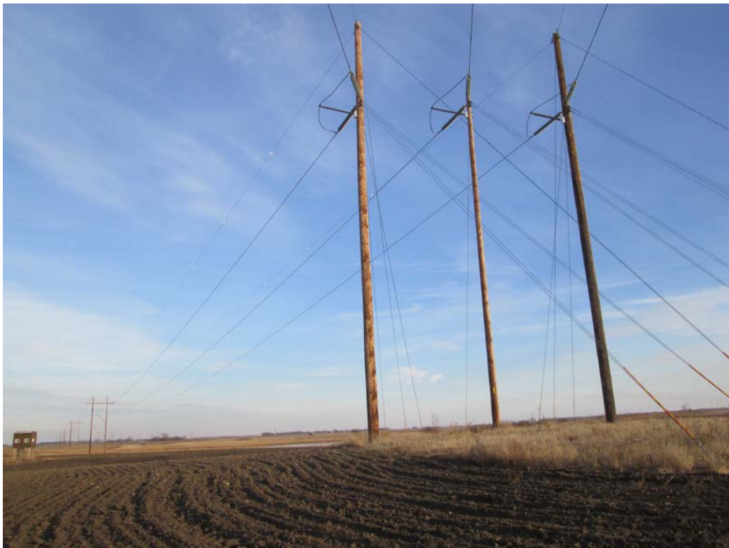
Below: Photo 14 (Structure 562) – Triple pole structure with guy wires. Structure between agriculture field and wetland. Looking northeast.
