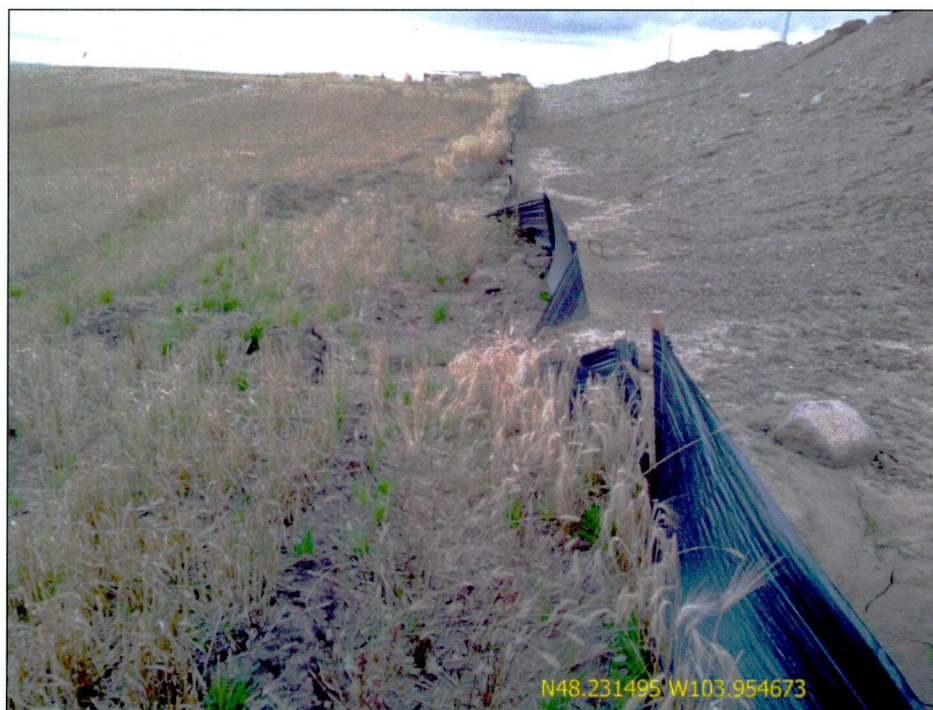
Figure 4. Recent activity on the soil storage piles and recent rain showers has filled the backside of the ECD. The silt fence effectively contained the soil subsidence. TIC committed to maintenance immediately.
