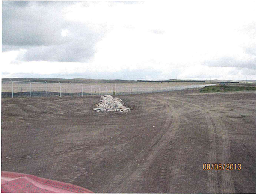
Figure 4. View from the northern edge of Garden Creek II looking east. Riprap installation to control drainage is seen.
