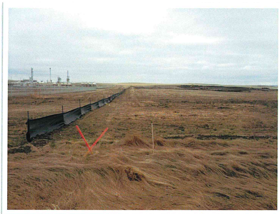
04/30/2013 Photo 2. View from southeast corner of GC III looking west. Silt fence installed on south property line.
