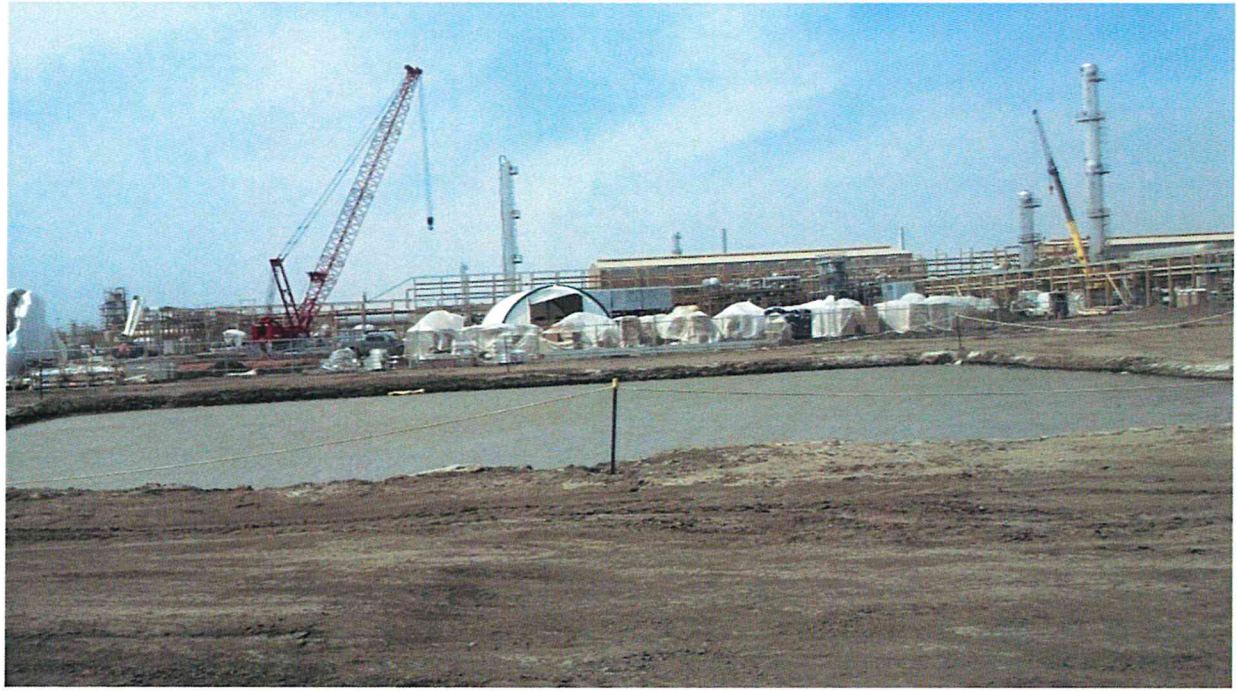
04/22/2014 Photo 15. View of a retention pond along the eastern edge of GC III looking west.
