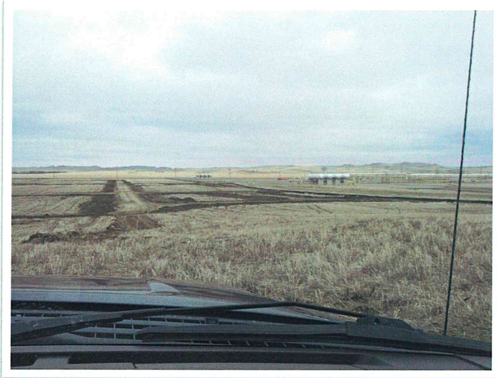
04/30/2013 Photo 3. View from west side of GC II looking east. Site roadways established and silt fence along southern boundary can be seen.
