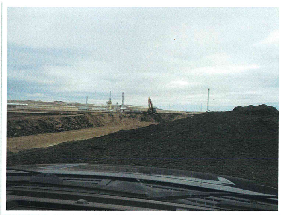
04/30/2013 Photo 4. View from the northwest corner of GC II looking south at the site grading efforts.
