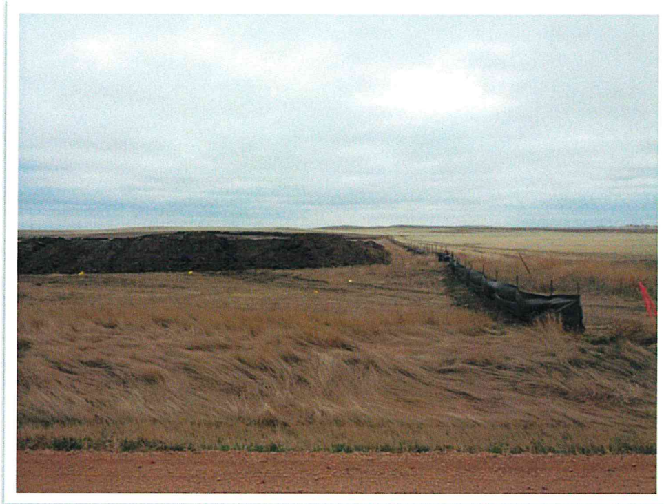
04/30/2013 Photo 1. View from northeast corner of GC III looking west. Silt fence installed on north property line.
