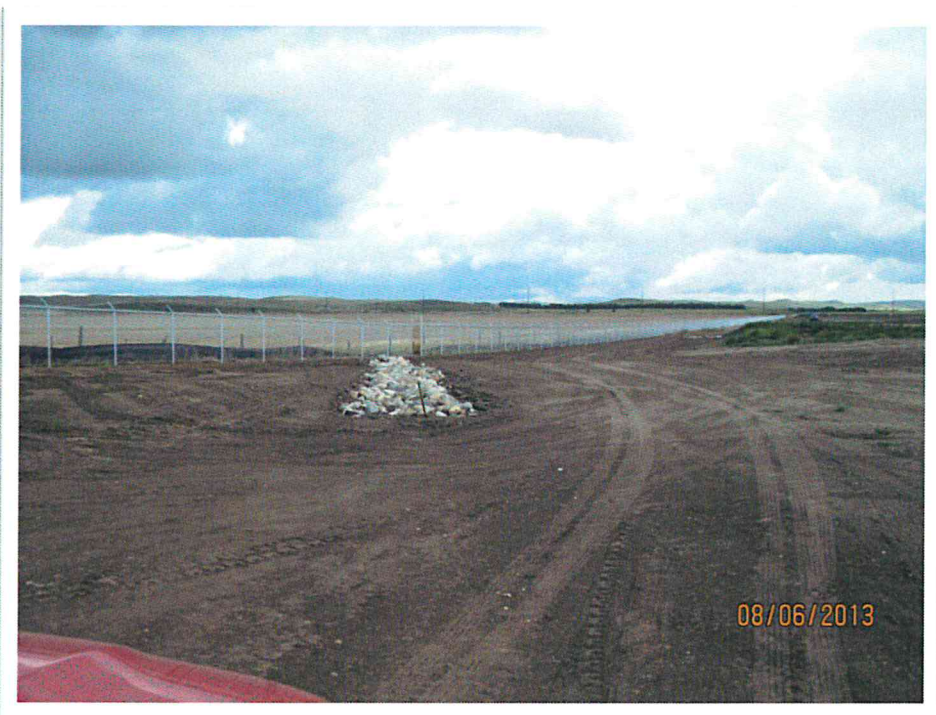
08/06/2013 Photo 8. View from the north edge of GC II looking east. Riprap installation to control drainage is seen.
