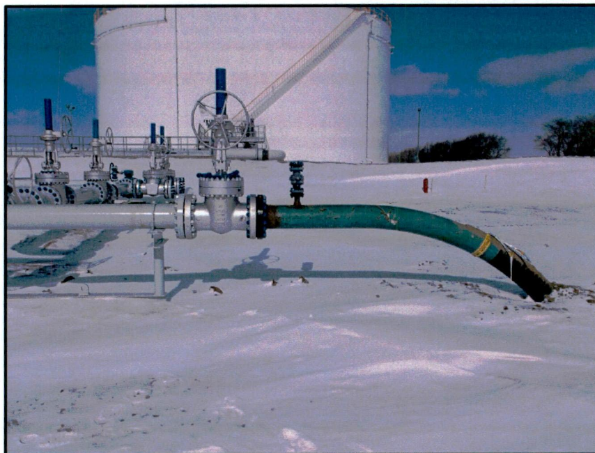
Photo 8. Direction: North. Tioga Rail Terminal pig launcher leading into transition area between RFT and TRT.
