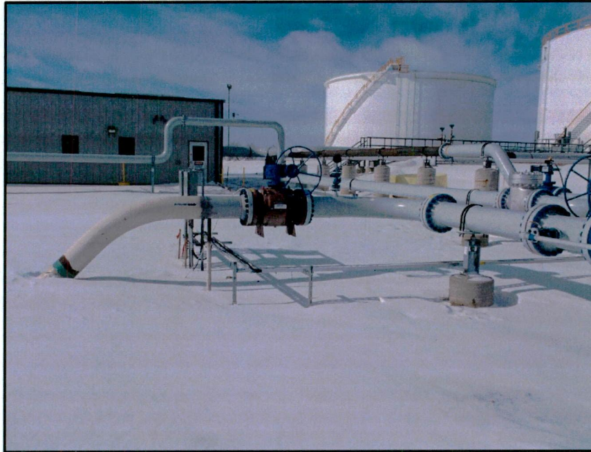
Photo 9. Direction: West. Ramberg Truck Facility pig launcher leading into transition area between RFT and TRT.
