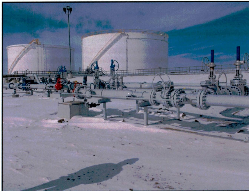
Photo 7. Direction: Northwest. Rail terminal transition area with between TRT and RFT, located on the north end of the project at Tioga Rail Terminal.
