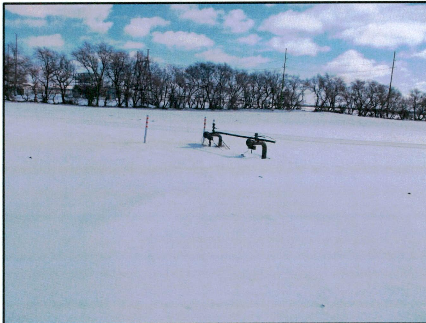
Photo 2. Direction: East. One of the pipeline markers that outlines transition point from existing to new pipeline running north to south, leading to Tioga Rail Terminal. East to west existing pipeline connecting to Ramberg Truck Facility.
