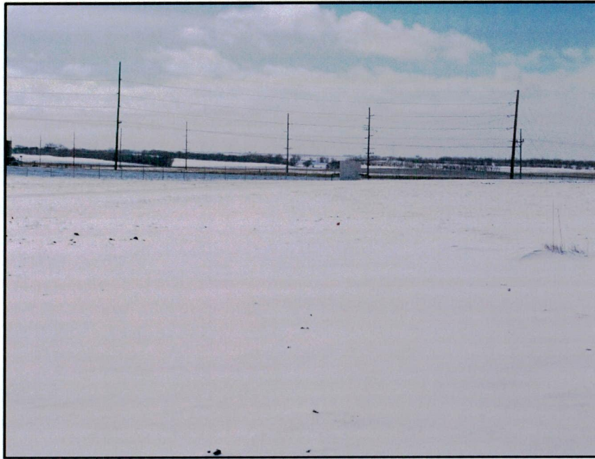
Photo 3. Direction: South. Area where existing pipeline ties into the Tioga Rail Terminal on the north end of the Project. The area still needs to be graded, compacted, and reseeded.
