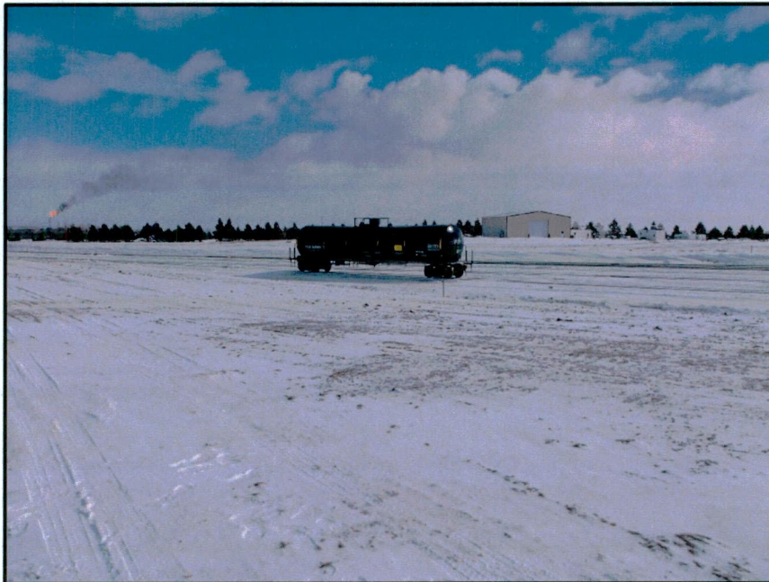
Photo 10. Direction: Southwest. Existing pipeline ROW area running north and south that connects tie in point shown in photo 1 and Tioga Rail Terminal, that still needs grading, compaction, and seeding.
