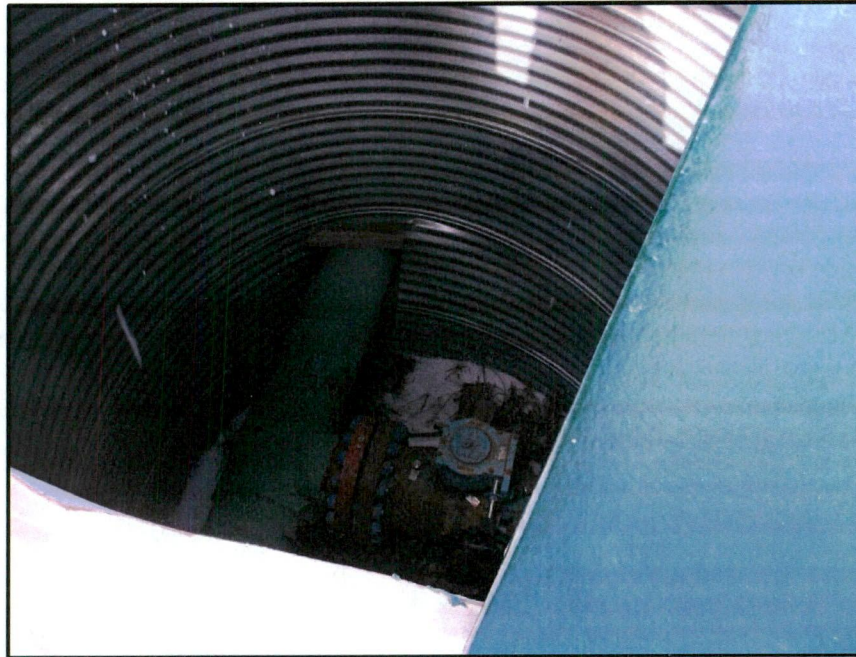
Photo 1. Direction: North. Inside protective container around transition between existing and new pipeline, located directly south of Tioga Rail Terminal.
