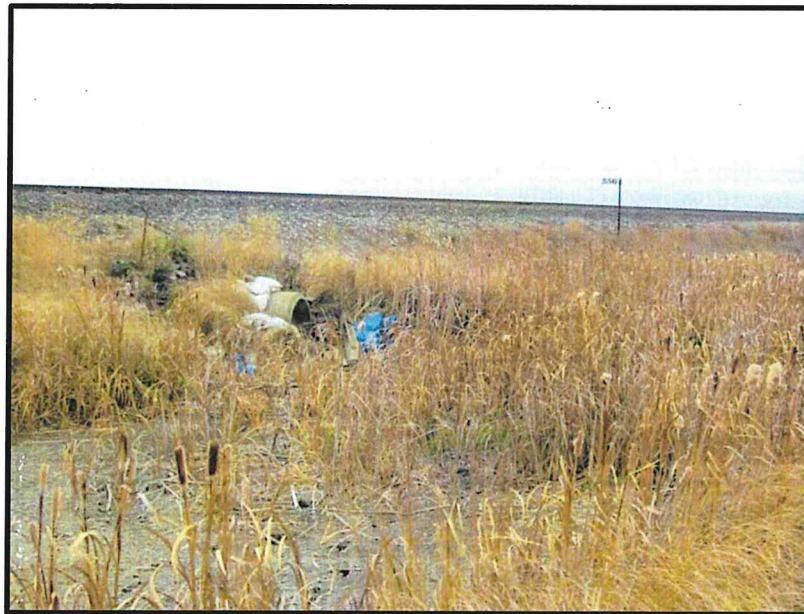
Photo 22. Direction: Southwest. Stream 24. Note the culvert allowing water movement under the railroad tracks.
