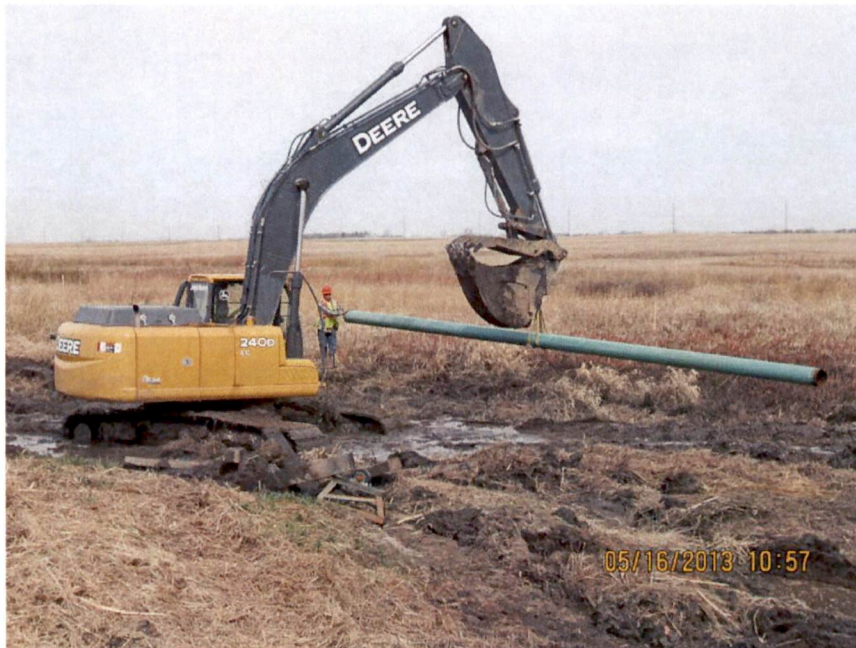
Photo: 4: No erosion or sediment control devices in place to protect wetland in the background.
