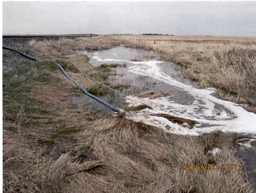
Photo: 6: Water being discharged to wetland without use of filtration or energy dissipation to prevent sediment from entering waterway, scouring or erosion.
