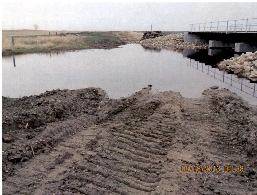
Photo: 2: Pipeline installation was done via HDD, equipment travel appears to have occurred through waterway without the placement/ use of erosion/sediment control measure to protect waterway. Also stabilization of disturbed banks has not been initiated.
