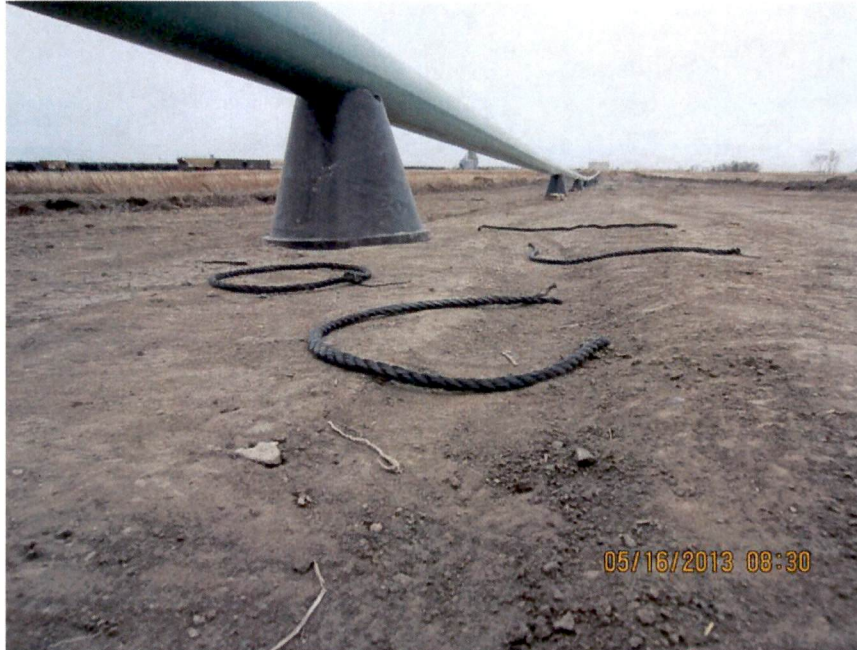
Photo: 1: Construction Debris on ROW
