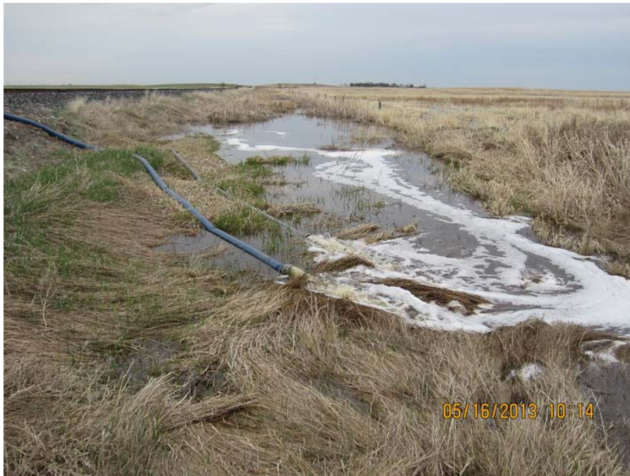
Photo: 6: Water being discharged to wetland without use of filtration or energy dissipation to prevent sediment from entering waterway, scouring or erosion.
