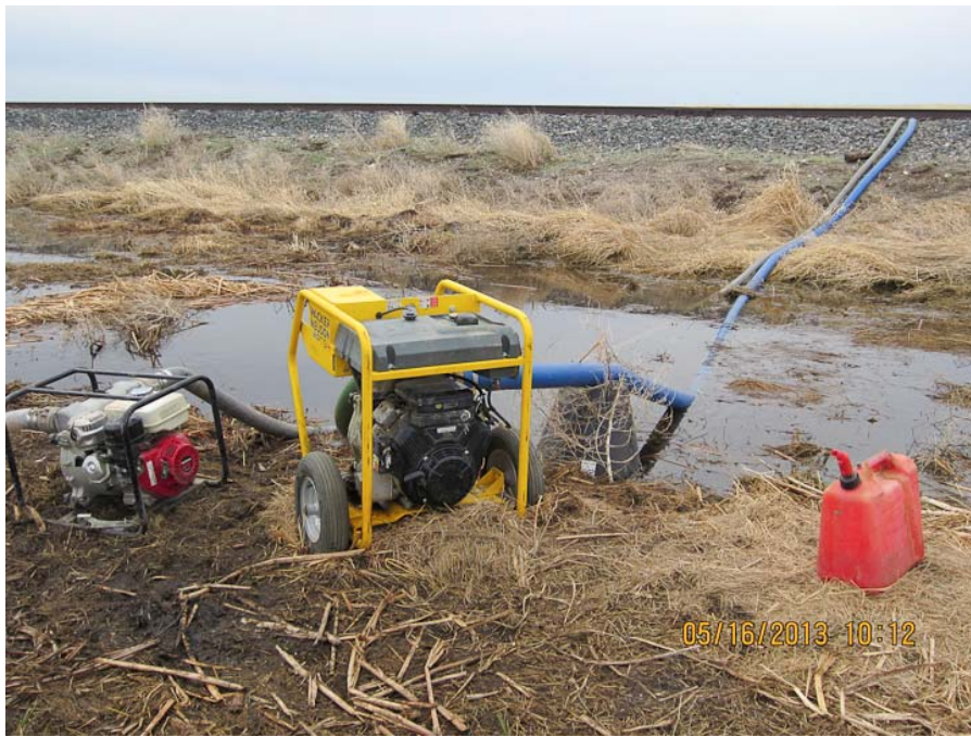
Photo: 5: Use of pumps and gas can within mapped wetland; no secondary containment or spill measures in place. Taken to the east of 89 th Ave. NW where pumping activities were occurring at time of inspection.
