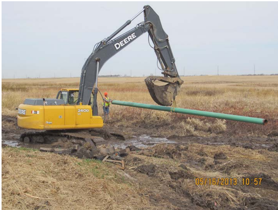
Photo: 4: No erosion or sediment control devices in place to protect wetland in the background.
