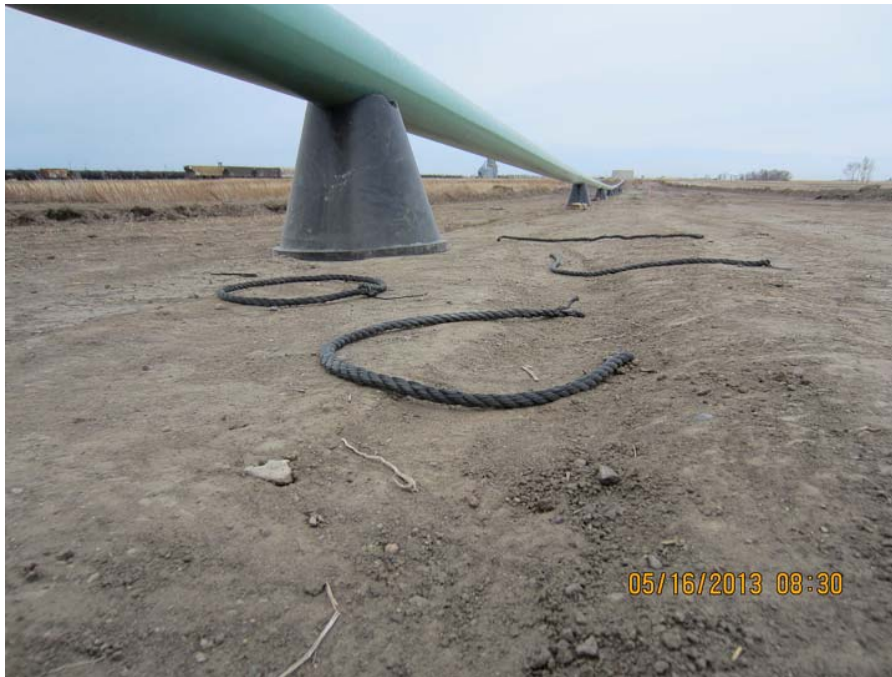
Photo: 1: Construction Debris on ROW
