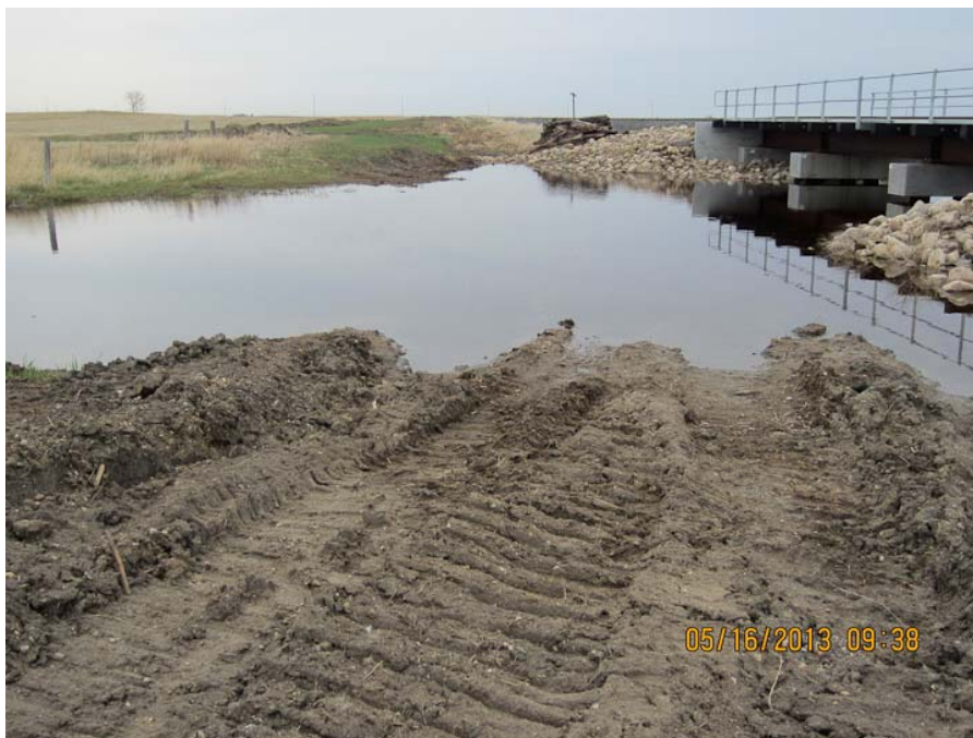
Photo: 2: Pipeline installation was done via HDD, equipment travel appears to have occurred through waterway without the placement/ use of erosion/sediment control measure to protect waterway. Also stabilization of disturbed banks has not been initiated.
