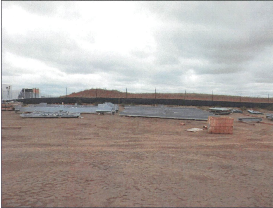
Figure 3. Photo taken from within the temporary construction site facing the south perimeter fence. Silt fencing was installed and working effectively around the site.
