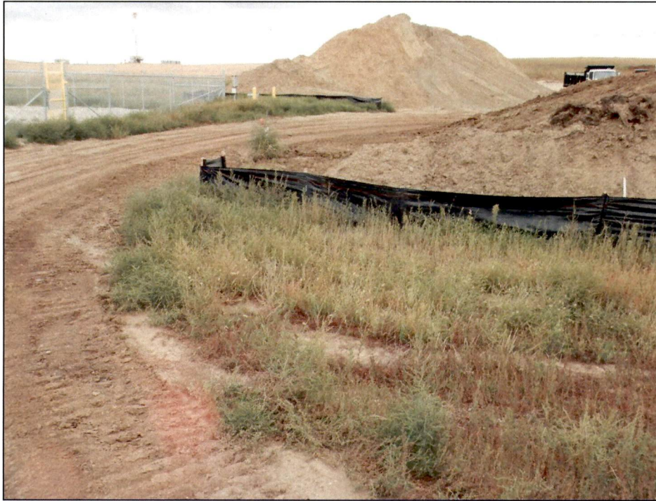
Figure 5. Photo of the northeast corner of the temporary construction site and soil storage piles. Silt fencing is in place and working properly to contain the soils on-site.
