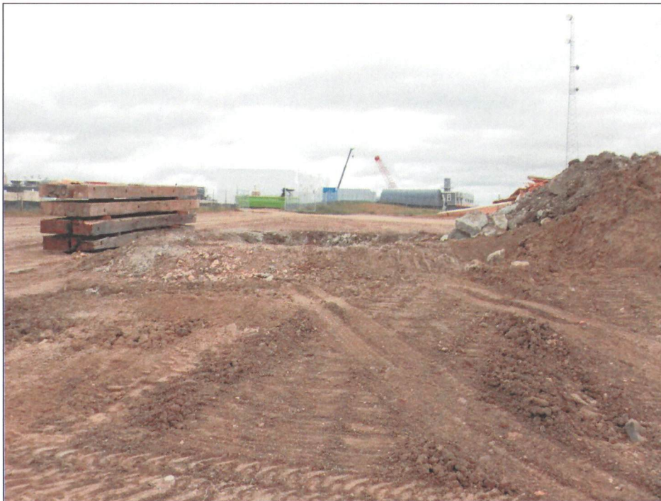
Figure 4. Concrete washout area. The basin was recently cleaned out and berms reconstructed.
