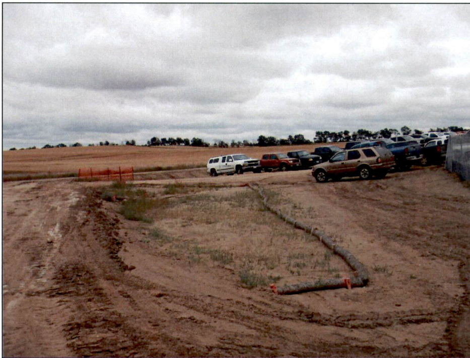
Figure 6. Straw wattles in place to reduce erosion of sandy soils into culvert.
