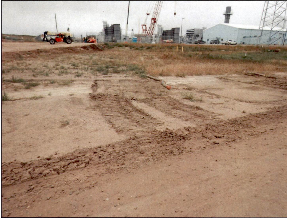
Figure 7. Straw waddles placed to contain sediments in a shallow ditch on-site. Sediment was recently removed from behind the waddles.
