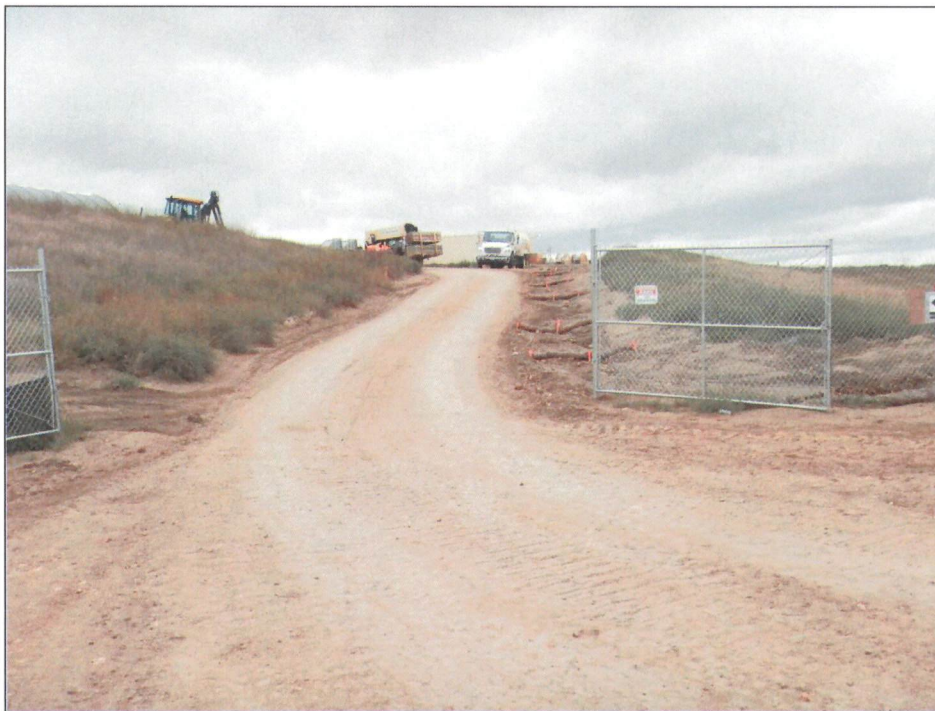
Figure 2. Photo of the access road to temporary construction site. Straw waddles are seen in shallow ditch which slow water flow and reduce soil erosion. Sediment from these ECD's are routinely cleaned out and repaired.
