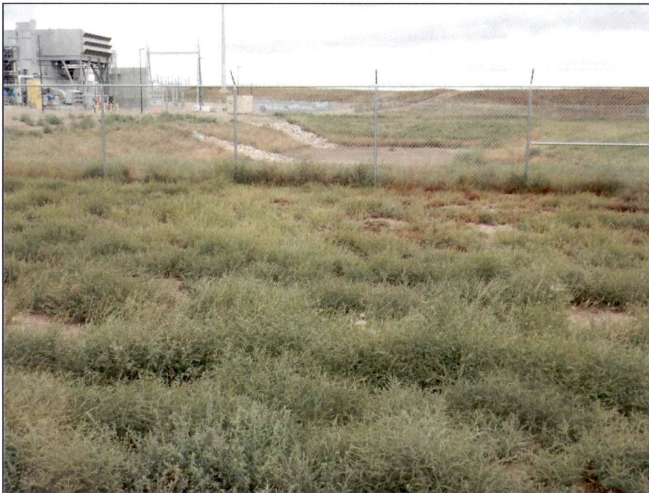
Figure 8. Permanent stormwater pond located west side of the permanent station. Inlets and outlets are rock rip-rapped and appeared to be in good condition. Any stored water has evaporated leaving a small amount of sediment in the bottom.
