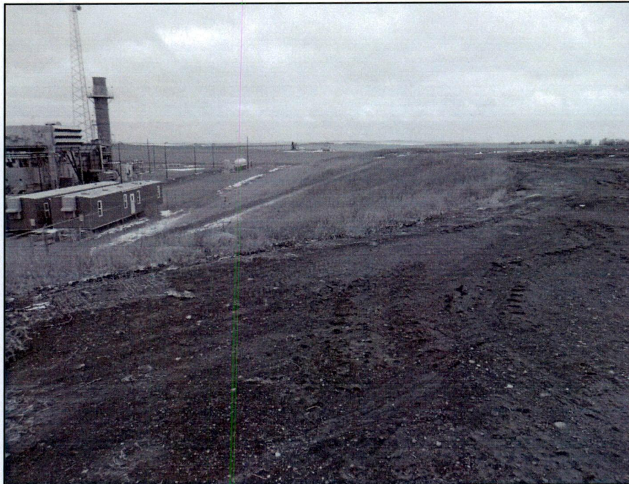
Figure 3. Photo looking north of the temporary construction laydown area (right). Gravel surface has been removed and topsoil replaced in December 2014. The area will be used again during construction of Phase III starting May 2015.
