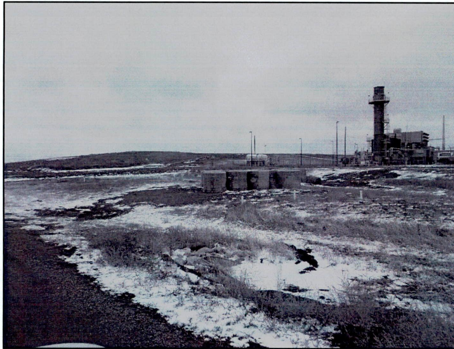
Figure 1. Photo from entrance road to the Lonesome Creek (LCS) Station looking southeast. Phase II construction (Unit 3) is visible to the right and the former temporary laydown area visible in background. Straw bales are to be used during reseeding efforts this spring.
