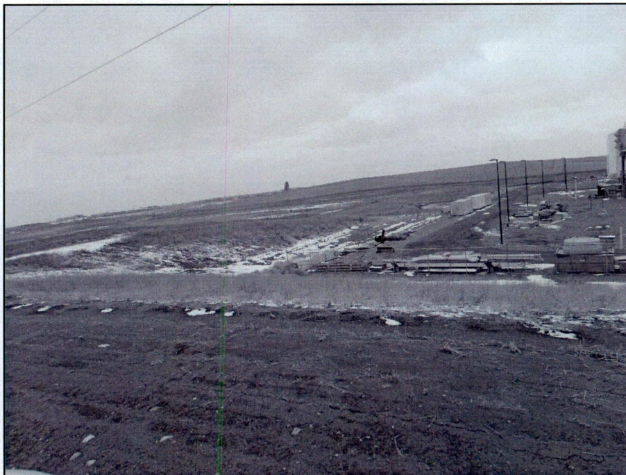
Figure 4. Overview looking north from the southwest corner of LCS. Erosion control matting in place on hillside and functioning from LCS Phase I construction. Weedy species will be mowed and sprayed as part of ongoing site maintenance.
