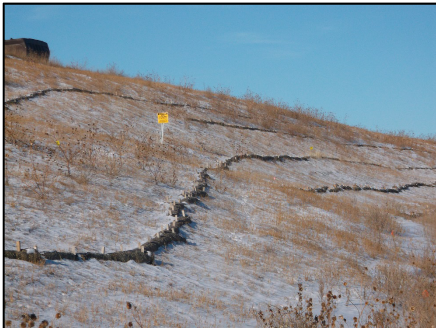
Photo 4. Direction: Northwest. Best Management Practices (BMP's) and above ground yellow pipeline marker are pictured above around the bend as the pipeline starts to head north parallel to County Road 15. The straw waddles will be removed in the spring; they were left in place to prevent erosion while vegetation was fully established.
