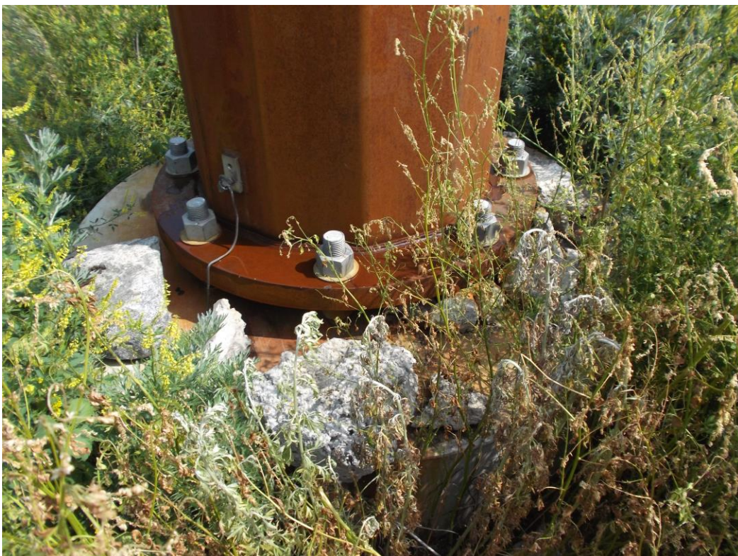
Below: Photo 12 (Structure 0685C) – Rocks and concrete waste set on structure base.
