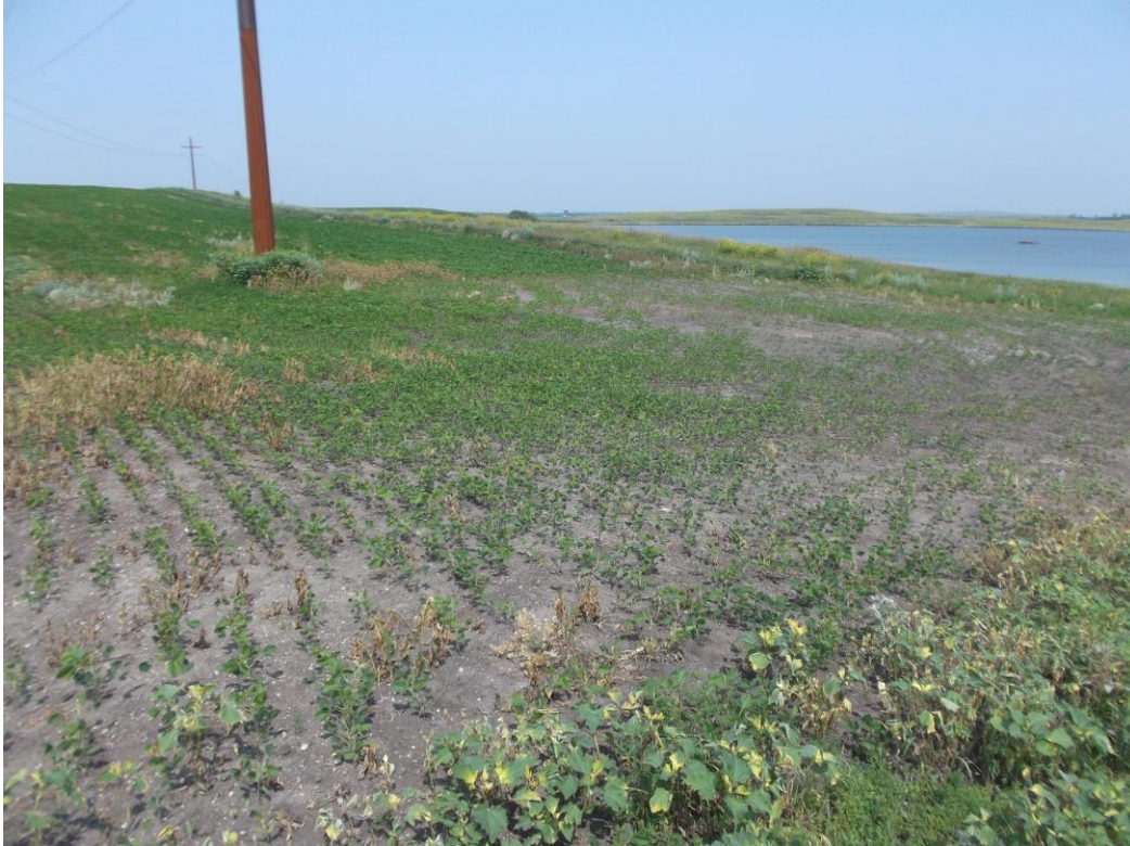
Above: Photo 11 (Observation Point 13) – Limited crop growth in low area near structure. Looking northwest.
