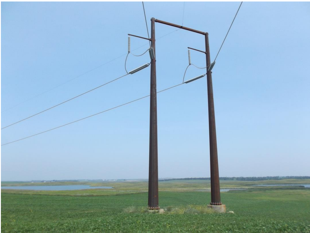
Below: Photo 6 (Observation Point 7) – Typical double pole structure at bend, where new alignment bends to avoid wetlands. Looking northwest.
