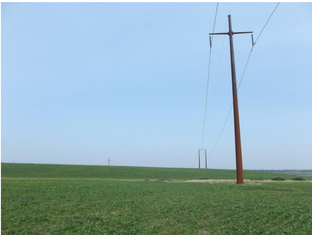
Below: Photo 2 (Observation Point 3) – First new structure at south end of project. Typical single pole structure. Looking northwest.
