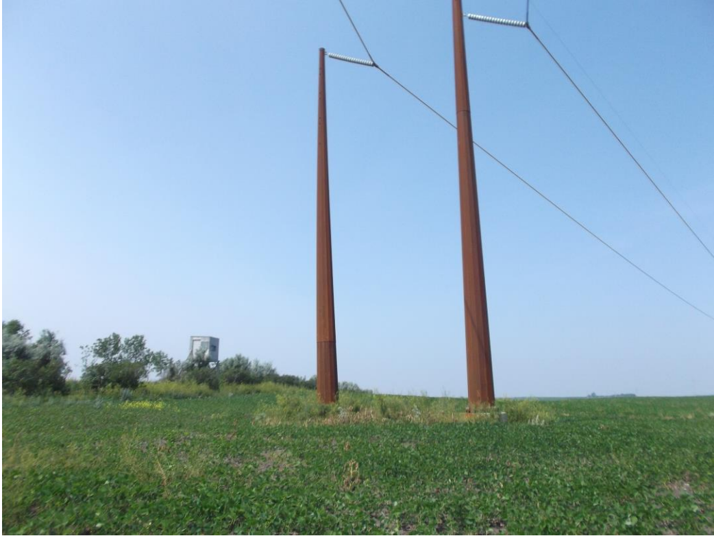
Above: Photo 17 (Observation Point 15) – Alternate double pole structure at bend. Looking west.
