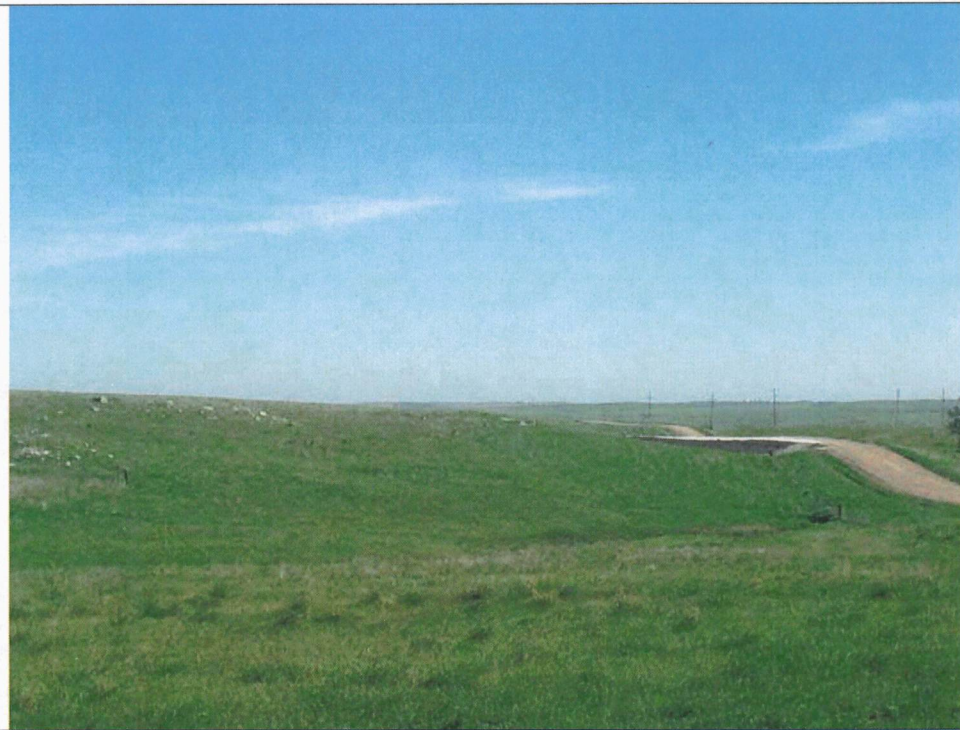
Photo 1: Access road for Turbine 463, from the south facing north. The staked archaeological / historic area can be seen in the foreground, and the access road construction avoids this identified area.
