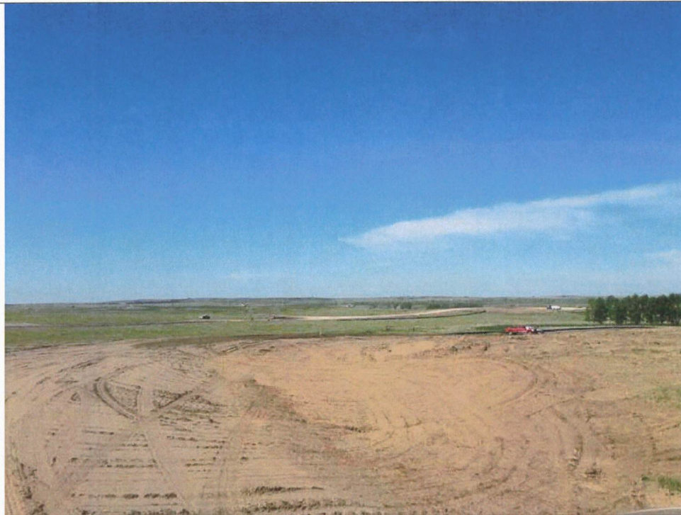
Photo 5: Access road and pad construction for turbines 452 (foreground) and 459 (background). Silt fencing observed.
