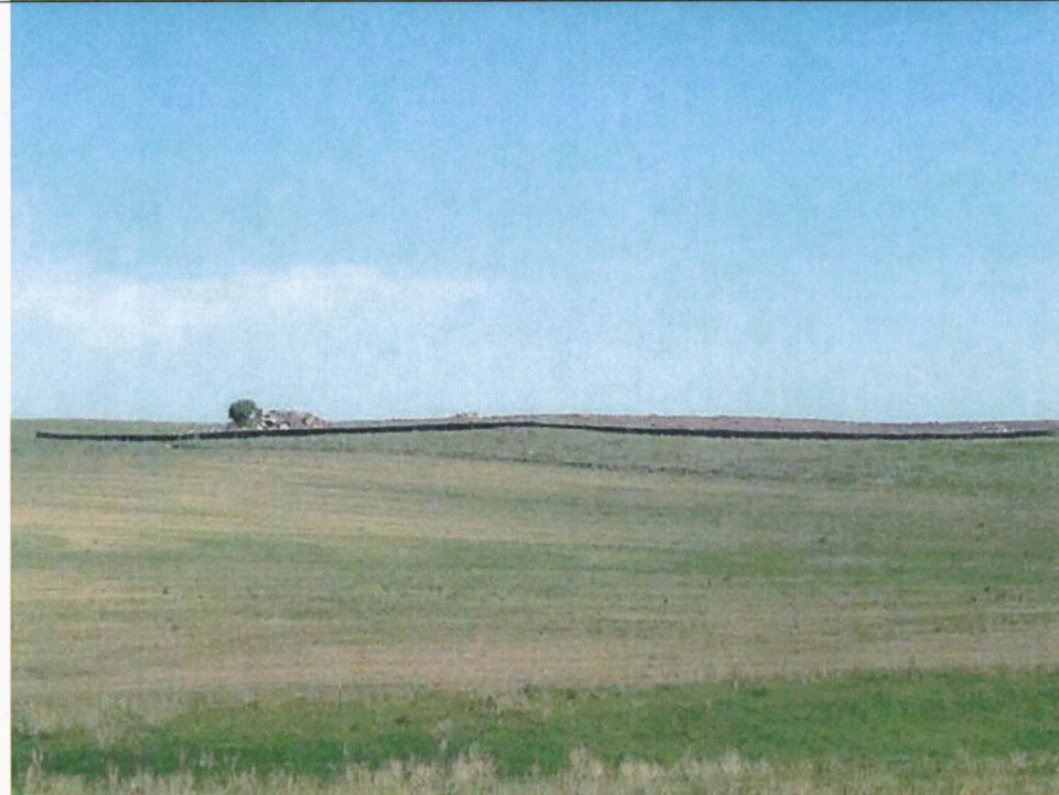
Photo 2: Silt fencing surrounding the pad for turbine 463. From the southeast facing northwest from 28 th street.
