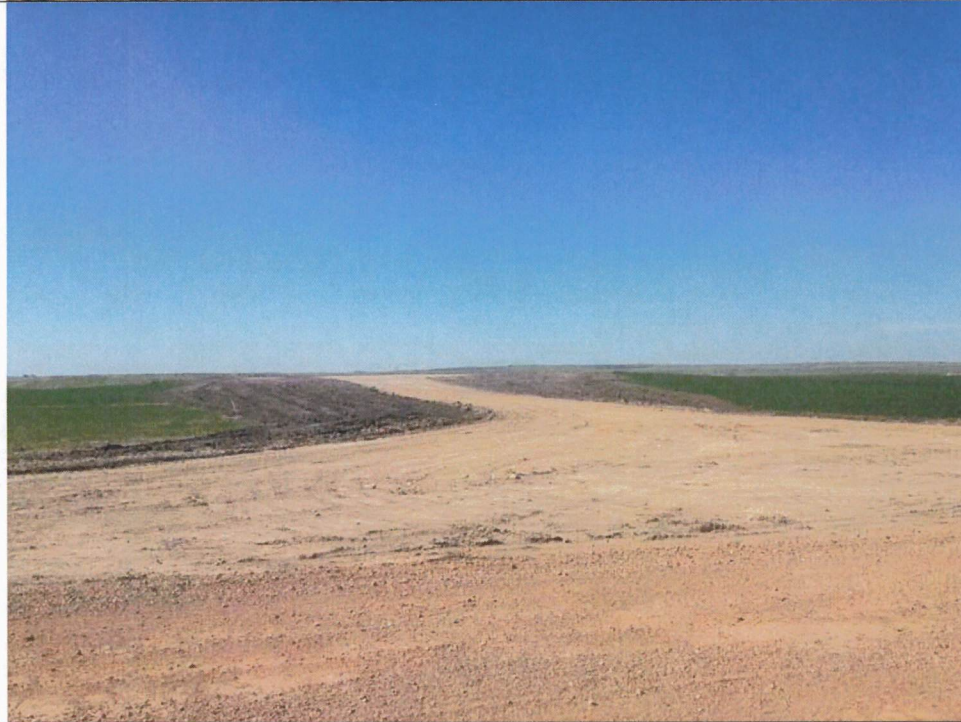
Photo 4: Access road (foreground) and pad (background) for turbine 461. Silt fencing was observed surrounding the pad.
