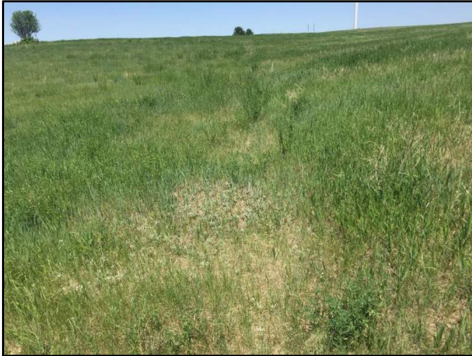
Photo 8. Facing: Northeast. Location: 47.019089, -101.706239 View of a soil ridge along the collector line southwest of T449. This ridge was likely formed from soil settlement after construction.
