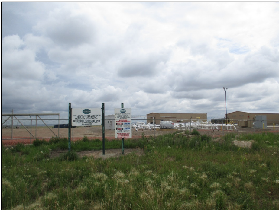
Photo 6. (GPS Point #17) – East Camp Creek Injection Station. Area is fenced and has signs. Direction: East.
