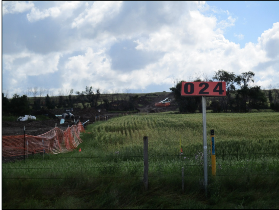
Photo 13. (GPS Point #30) – Pipeline ROW in crop land. Construction of a different pipeline is to the left of photo, paralleling part of Hiland’s Market Center pipeline. Direction: East.
