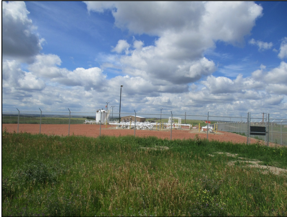
Photo 19. (GPS Point #37) – White Earth Booster Station. Direction: West.
