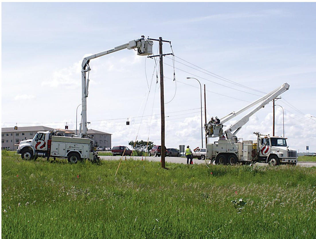
Submitted Photo Xcel Energy crews work on a electrical line in Minot.
