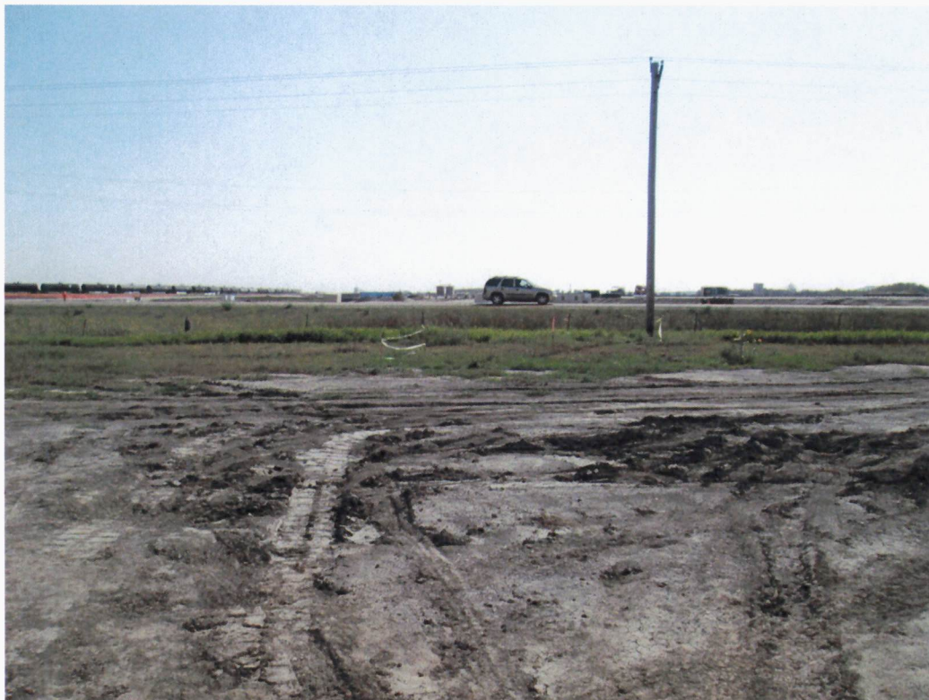
Below: Figure 2. Road Crossing, Bore hole fenced off with tape
