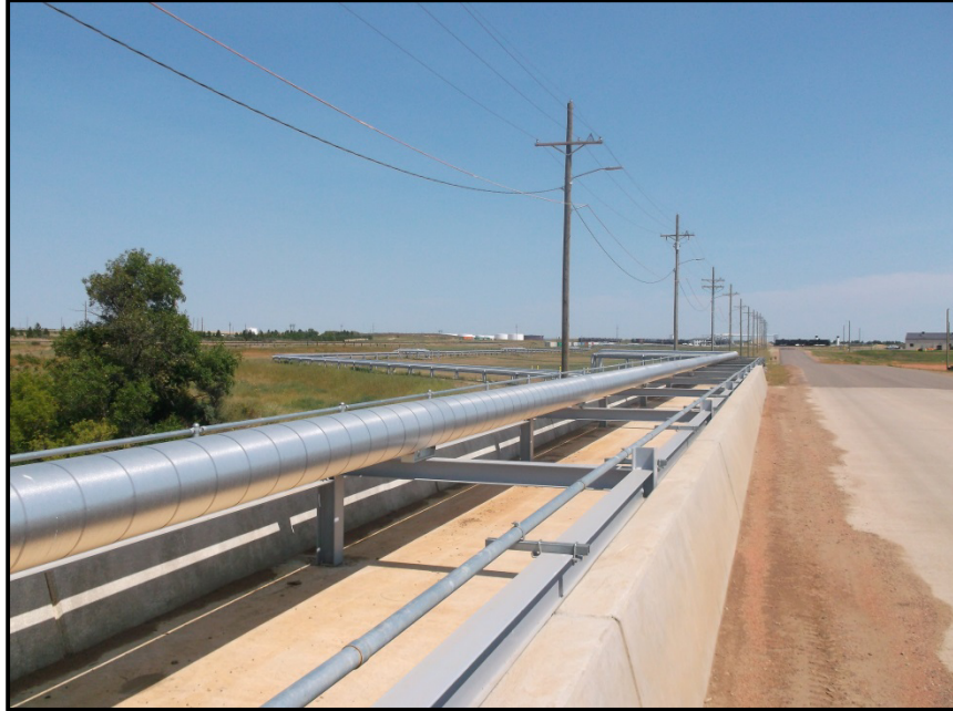
Photo 15. Direction: East. Pipeline running east and west, crossing the Heart River along a bridge. While installing the pipeline damage was done to the bridge or roadway as depicted above. (This photo is from the second and final inspection of the pipeline).
