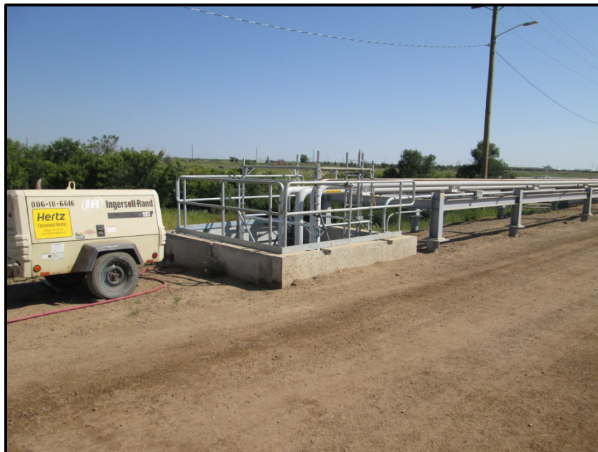
Photo 4. Direction: Northeast. Vertical entrance point of pipeline where it bends south, parallel to the Heart River and underneath the facility access road.
