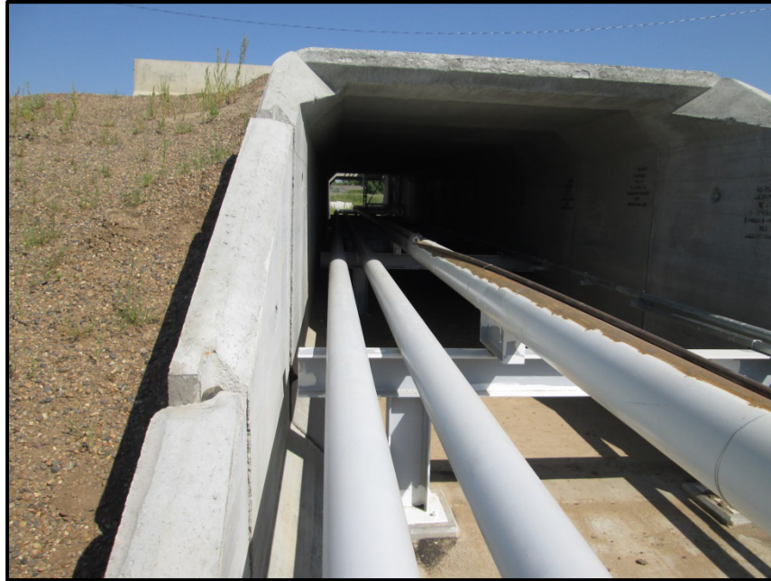
Photo 3. Direction: North. View of the pipeline section that runs through the box culvert underneath the facility access road. Preventative spill/leak containment measures taken are depicted in the photo above as well.
