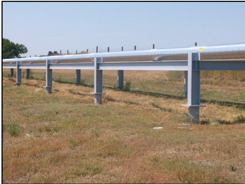
Photo 14. Direction: Northwest. Depicted above is an example of the recovery of the ROW to preconstruction conditions. (This photo is from the second and final inspection of the pipeline).
