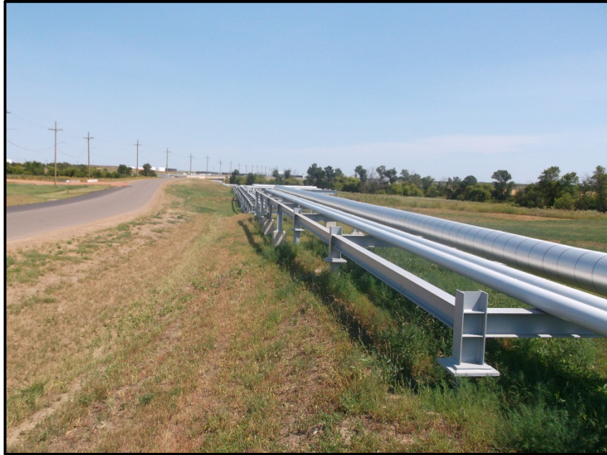
Photo 17. Direction: East. Depicted above is an example of the recovery of the ROW to preconstruction conditions. This section of the pipeline is south of the facility access road running east to west. (This photo is from the second and final inspection of the pipeline).
