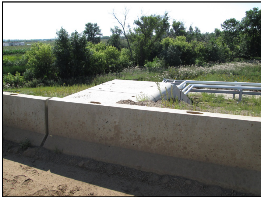
Photo 2. Direction: Southeast. Pipeline entering underground box culvert beneath the facility access road and running parallel to the Heart River.
