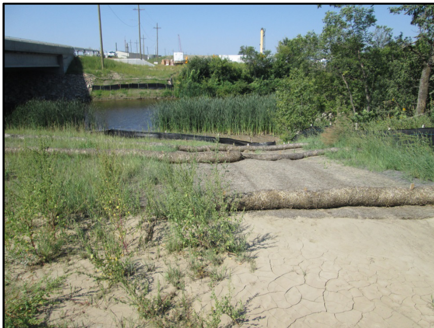
Photo 6. Direction: East. Erosion control measures and BMP's (Best Management Practices) in place along bridge and pipeline crossing the Heart River.
