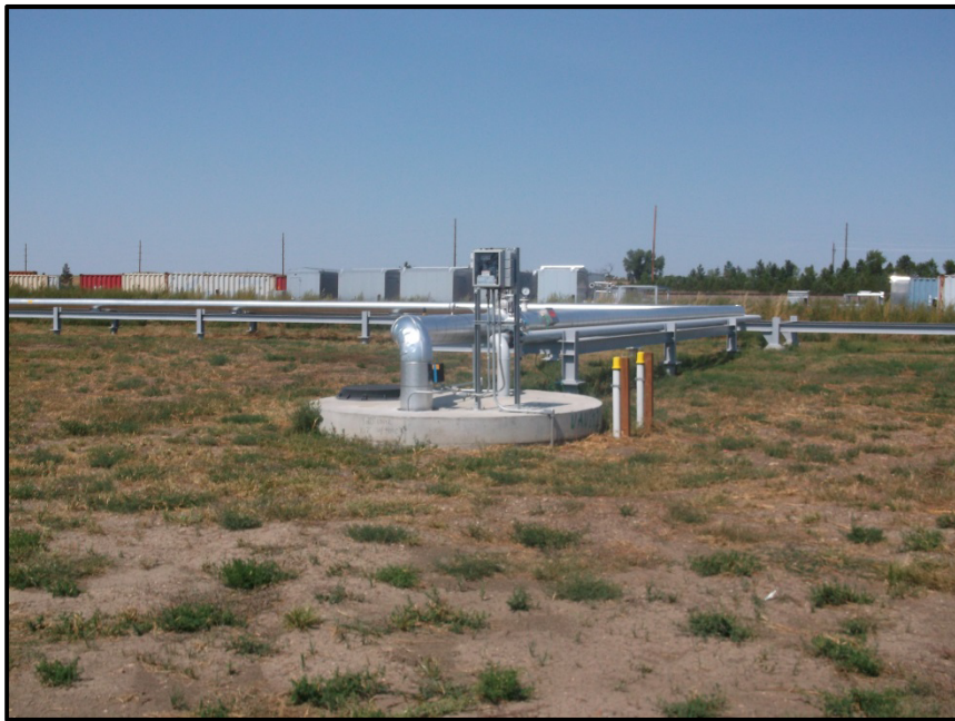
Photo 10. Direction: Northwest. Pictured above is the pipeline bending to the south prior to boring under 116 th Ave SW and entering underground structure. (This photo is from the second and final inspection of the pipeline).
