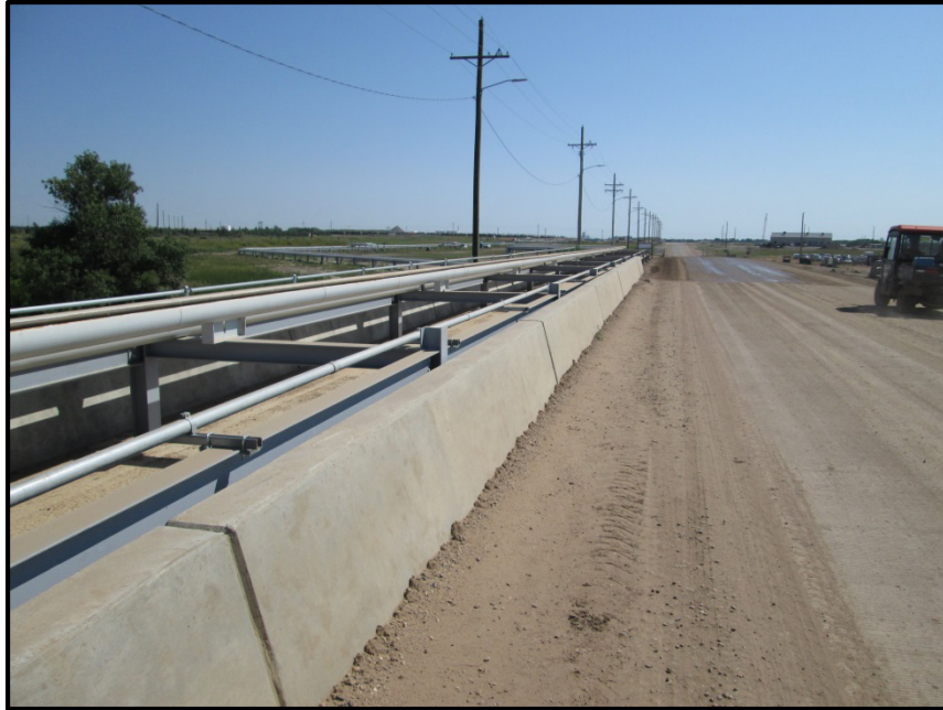
Photo 5. Direction: East. Pipeline running east and west, crossing the Heart River along a bridge. While installing the pipeline damage was done to the bridge or roadway as depicted above.
