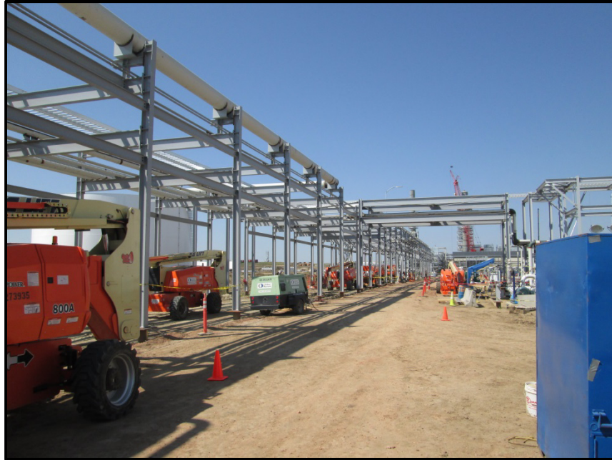
Photo 1. Direction: Northwest. Pipeline leaving the Dakota Prairie Refinery and under construction in the photo.
