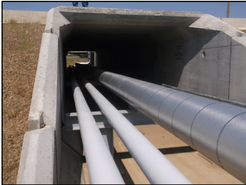
Photo 16. Direction: North. View of the insulated pipeline section that runs through the box culvert underneath the facility access road. Preventative spill/leak containment measures taken are depicted in the photo above as well. (This photo is from the second and final inspection of the pipeline).
