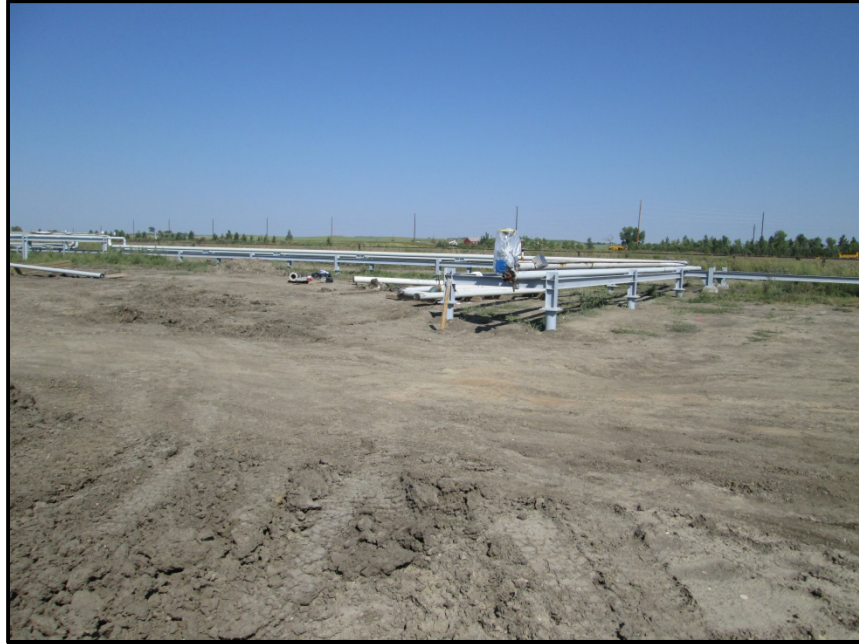
Photo 9. Direction: Northwest. Termination of the Pipeline prior to boring under 116 th Ave SW.
