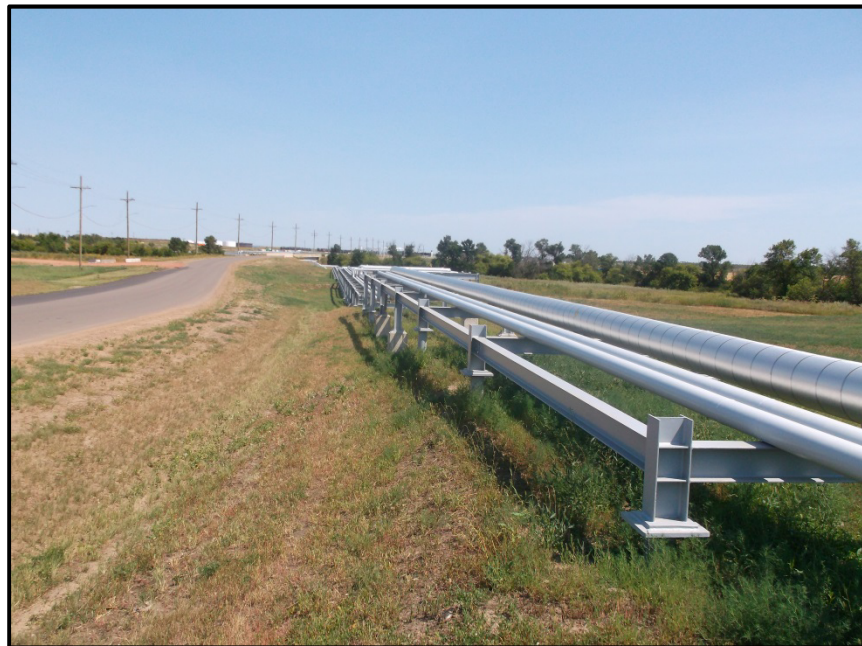
Photo 12. Direction: West. Completed pipeline with 8" line insulated and heat traced, ROW returned to pre-construction conditions. (This photo is from the second and final inspection of the pipeline).
