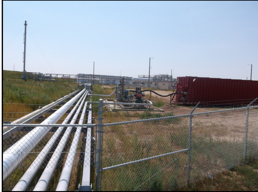
Photo 13. Direction: Southwest. The picture above depicts where the pipeline enters the Dakota Prairie Refinery, the security measures in place are also depicted. (This photo is from the second and final inspection of the pipeline).
