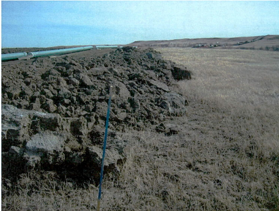
Photo 10 – Spoil Placed Outside of Identified Right-of-Way
