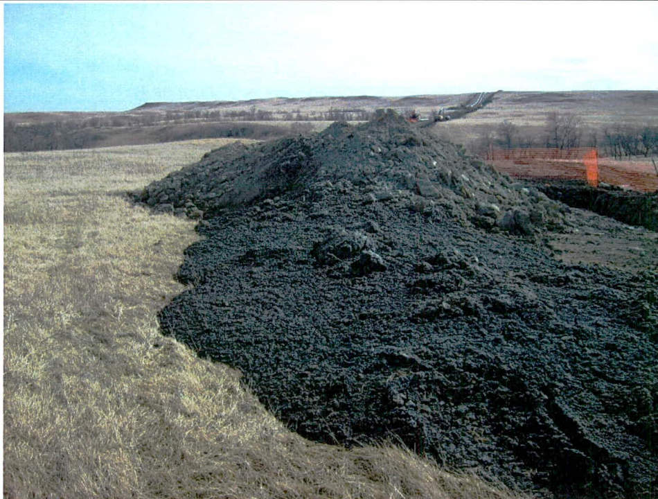
Photo 8 – HDD Spoil Pile with No Erosion Control Devices
