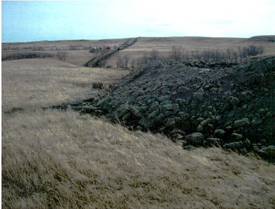
Photo 7 – HDD Spoil Pile with No Erosion Control Devices
