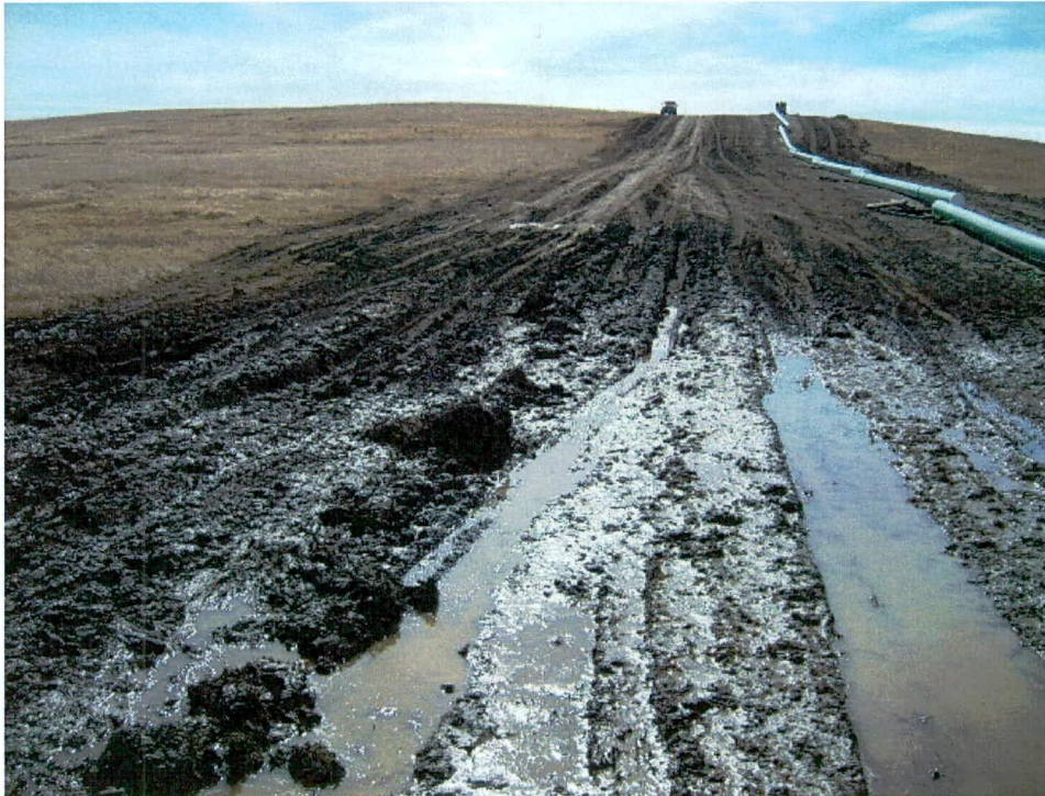
Photo 5 – Rutting Along the Right-of-Way
