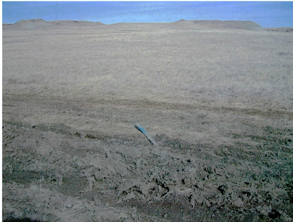
Photo 2 – Construction Staking to be Replaced
